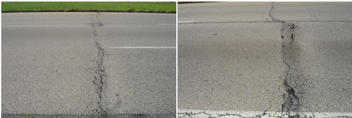
Figure 3 Typical Reflection Cracking in Composite Pavements
