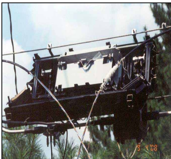
Figure 8-4: Aerial Fiber Optic Cable Splice Box - Photograph Courtesy Adesta, LLC
