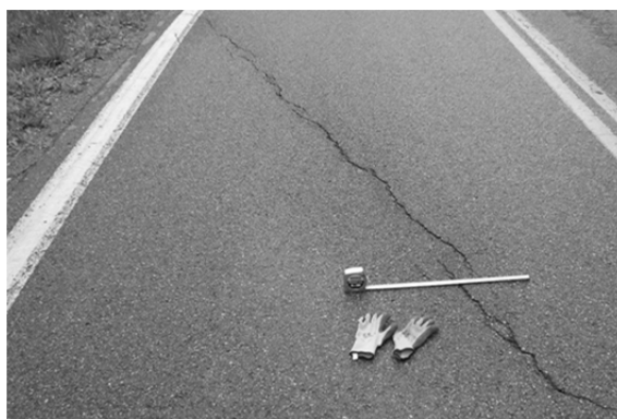
Figure 2.4. Pavement crack on SR 690 at 4.6 miles northbound.
