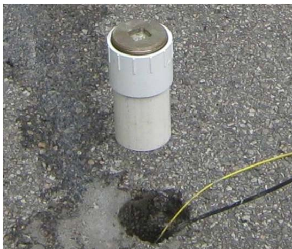
Figure 2.11. PVC tube with a screw cap to protect additional cable from damage.
