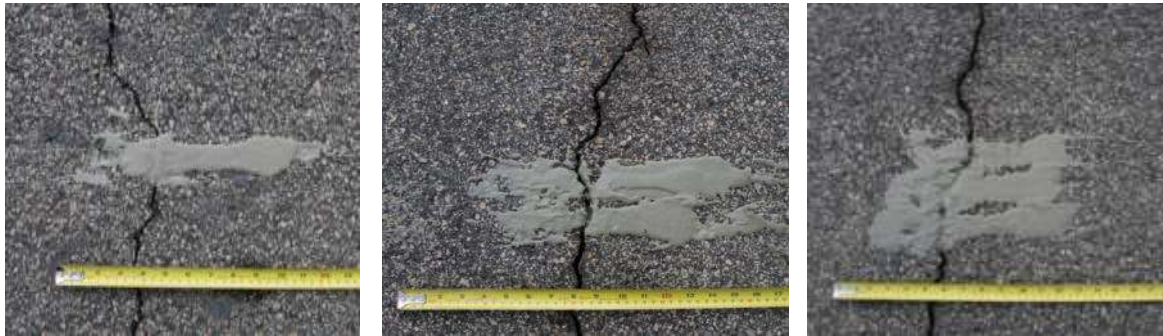
Figure 13. Examples of Sealant Dispensed In Pavement Crack From System Parking Lot Tests
