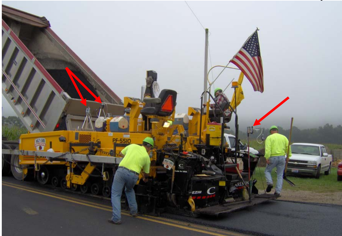
Photograph of the paving operation on SR541 showing monitoring equipment attached to paver, indicated with arrows.
