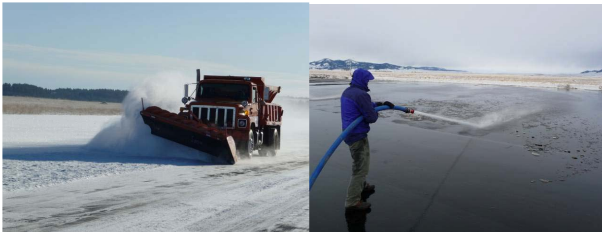
Figure 11 Clearing and washing test sections on the driving surface area using a plow truck and high pressure hose.
