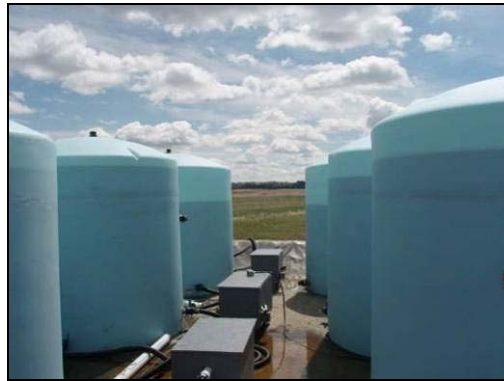
FIGURE 1 The six 3000-gallon tanks full of liquid deicers at TRANSEND. Along the center line are the three pumps used to mix one tank of each deicer.
