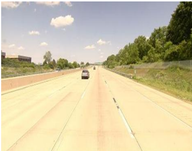
Figure 35: Overall Condition of SR 202 Segment 440 Northbound.
