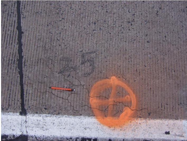
Figure 125: Digitally Enhanced Map-cracking of I 80 Segment 1914 Eastbound (Distressed Section)
