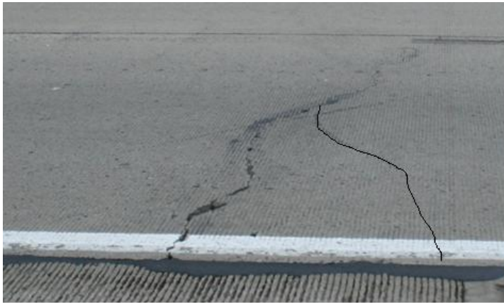
Figure 151: Medium Severity Transverse Crack with Digitally Enhanced Branching Drying Shrinkage Crack on I 80 Segment 1914 (Distressed Section)
