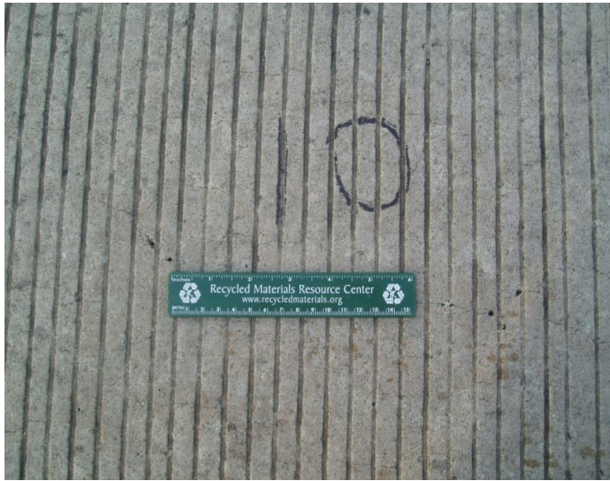
Figure 38: Close-up of Fine Microcracking of SR 202 Segment 440 Northbound, Slab 10.
