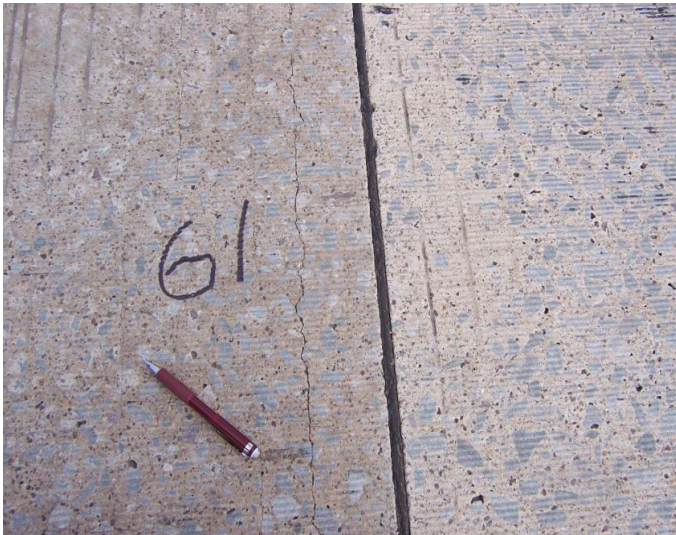
Figure 54: Joint Close-up of US-22Murrysville Segment 50 Eastbound, Slabs 61 and 62.
