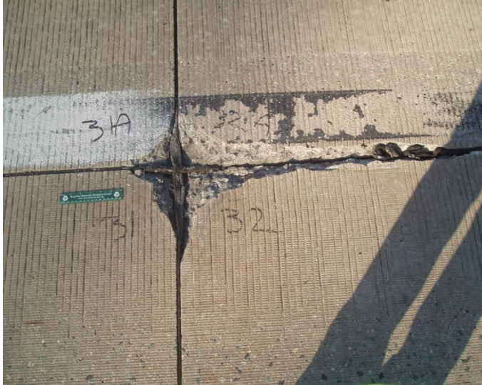
Figure 36: Joint Intersection between Adjacent Lanes of SR 202 Segment 440 Northbound Slabs 31 and 32.
