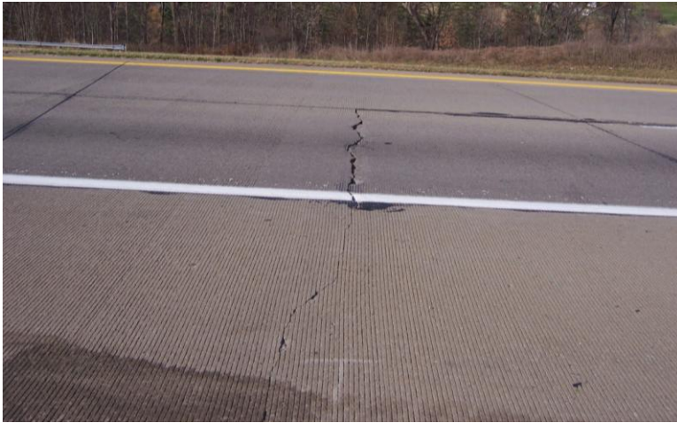
Figure 87: High Severity Transverse Crack of I 79 Segment 470 Northbound (Distressed Section)
