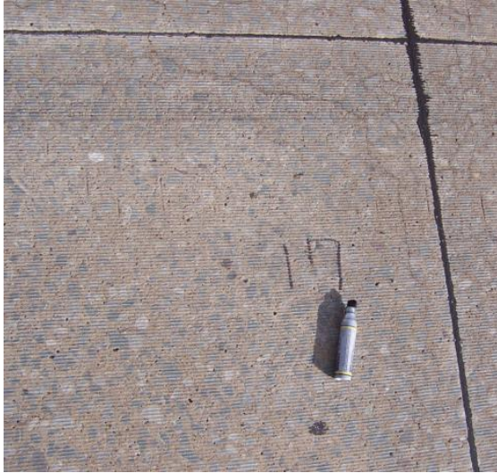
Figure 63: Map Cracking Observed on Slab 17 US 22, Westmoreland County Segment 50 Eastbound
