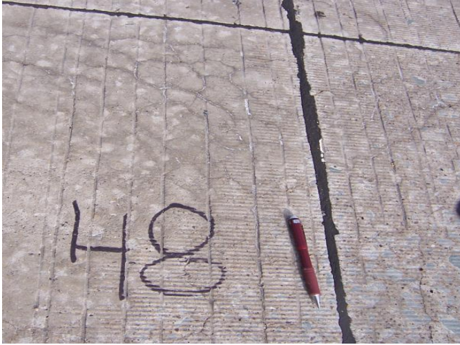
Figure 52: Joint Close-up of US-22 Murrysville Segment 50 Eastbound Slabs 48 and 49.
