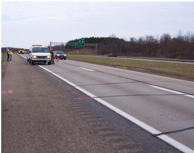
Figure 4: Overall Condition of SR 60 Segment 323 Southbound (Distressed Section)
