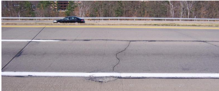
Figure 88: Digitally Enhanced Low Severity Transverse Crack and an Asphalt Patch of I 79 Segment 470 Northbound (Distressed Section)
