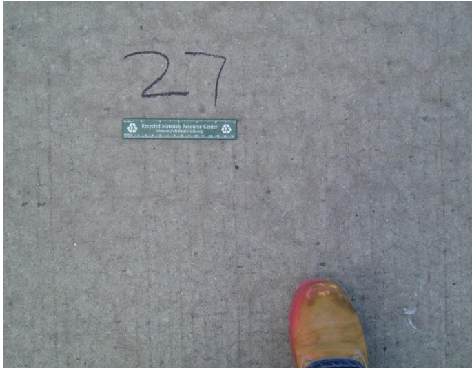
Figure 39: Close-up of Microcracking of SR 202 Segment 440 Northbound, Slab 27.
