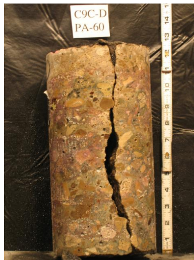
Figure 20: High Severity Transverse Crack Core of SR 60 Segment 323 Southbound Slab 9 (Distressed Section)
