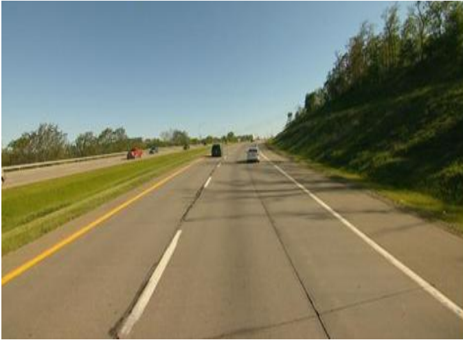
Figure 83: Overall Condition of I 79 Segment 470 Northbound (Distressed Section)
