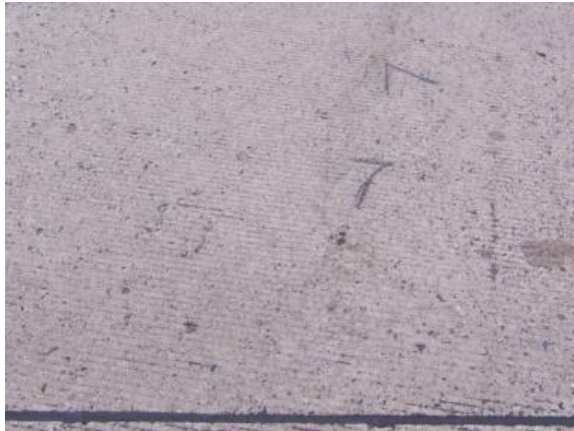
Figure 124: Longitudinal Crack of I 80 Segment 1914 Eastbound (Distressed Section)
