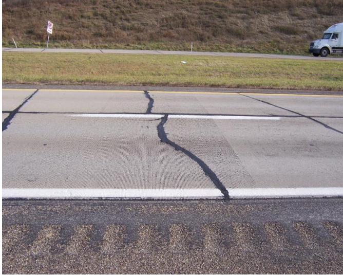
Figure 6: Mid-slab Transverse Cracking for SR 60 Segment 323 Southbound, Slab 5 (Distressed section).
