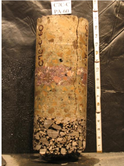
Figure 21: Low Severity Transverse Crack Core of SR 60 Segment 303 Southbound Slab 7 (Control Section).
