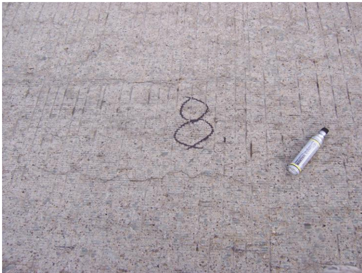
Figure 53: Slab Close up of Midslab Longitudinal Cracking from US-22 Murrysville Segment 50 Eastbound, Slab 8.
