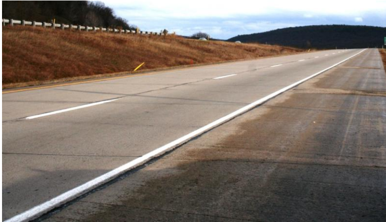
Figure 119: Overall Condition of I 80 Segment 1914 (Portion of Distressed Section)
