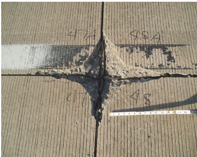
Figure 37: Joint Intersection between Adjacent Lanes of SR 202 Segment 440 Northbound Slabs 47 and 48.
