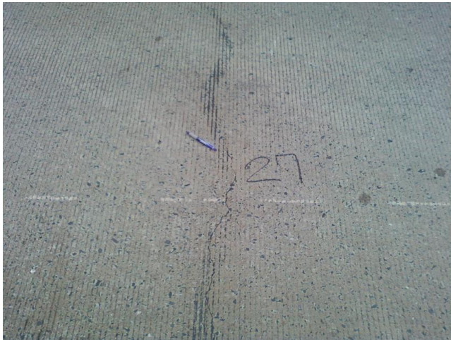
Figure 122: Low Severity Transverse Crack of I 80 Segment 1914 Eastbound (Distressed Section)
