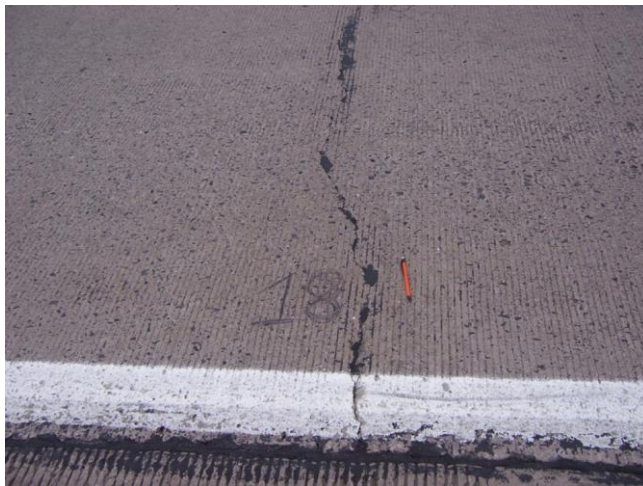
Figure 123: Medium Severity Transverse Crack of I 80 Segment 1914 Eastbound (Distressed Section)
