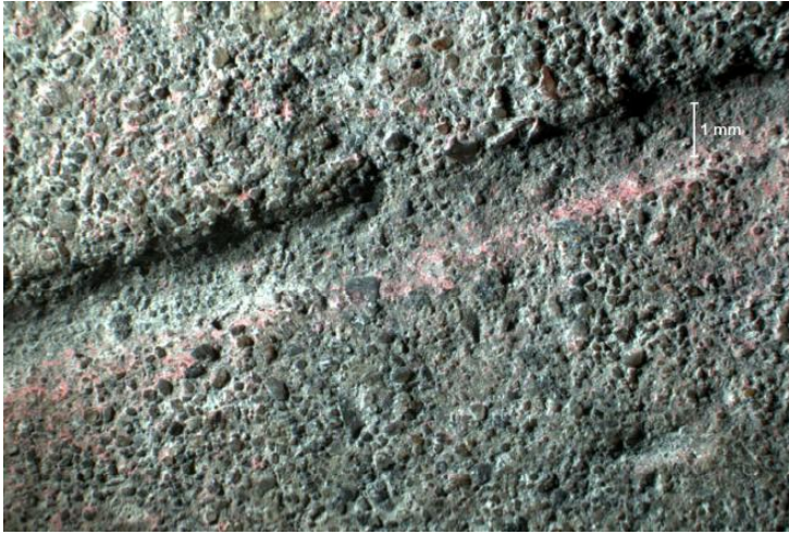
Figure 65: Wear/Erosion of the Pavement Surface as Seen on the Surface of Core C34-MS22.
