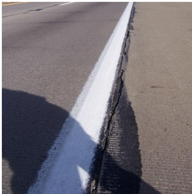
Figure 86: Lane-to-Shoulder Joint of I 79 Segment 470 Northbound (Distressed Section)
