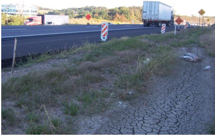
Figure 91: Typical Ponding Area of I 79 Segment 470 Northbound (Distressed Section) (photo taken after overlay placement)
