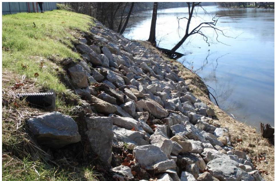
Figure 5.35: A Picture Showing the Rip Rap Placed at the Toe of the Restored Slope at MRG-376 Site
