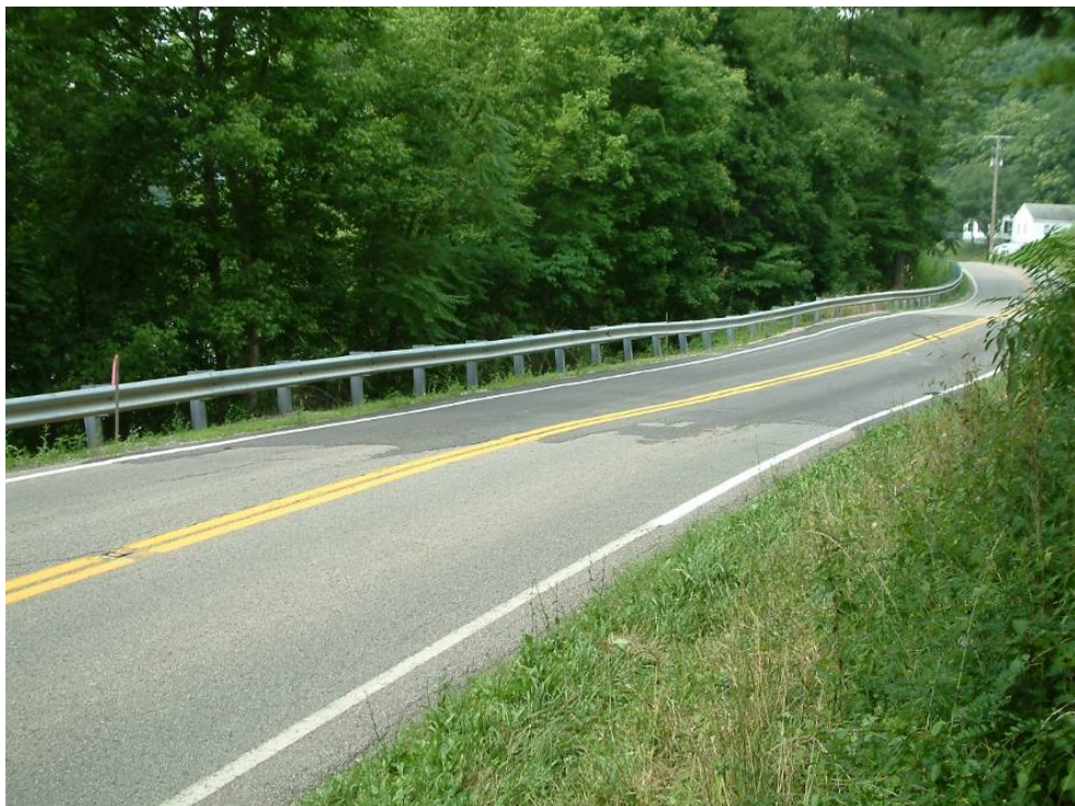
Figure 5.33: A Picture Showing MRG-376 Site before Slope Repair
