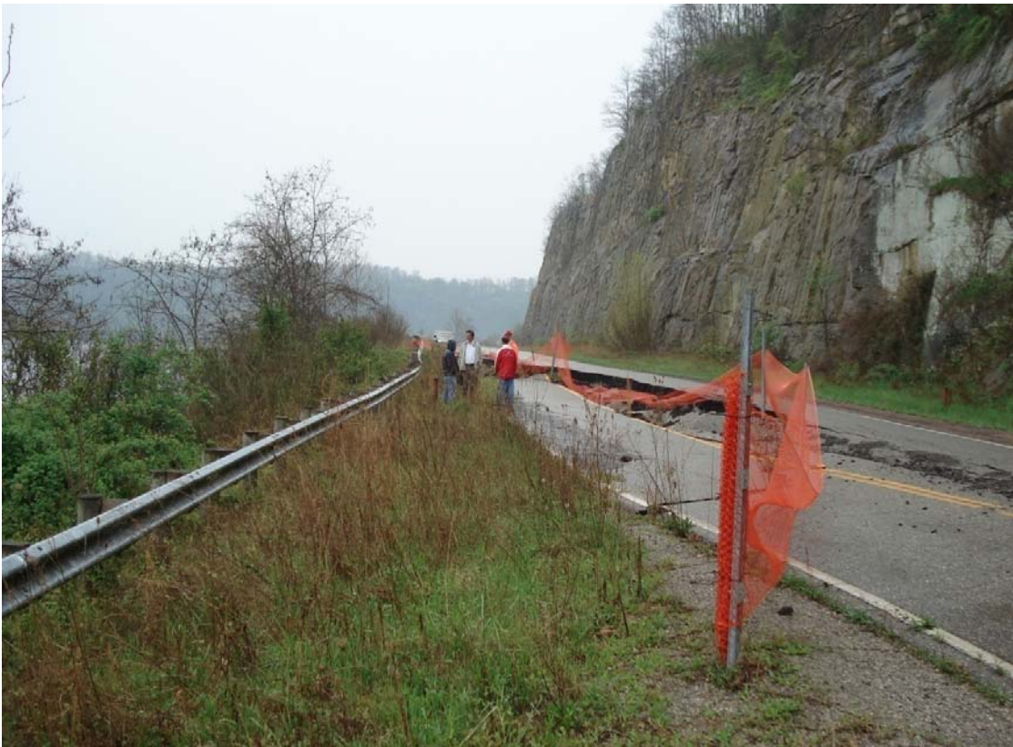
Figure 4.13: A Picture Showing the ATH Site Condition Prior to Construction of Test Drilled Shafts
