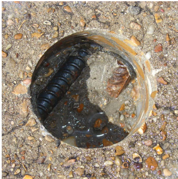
Figure 6 Partial depth core showing little steel corrosion
