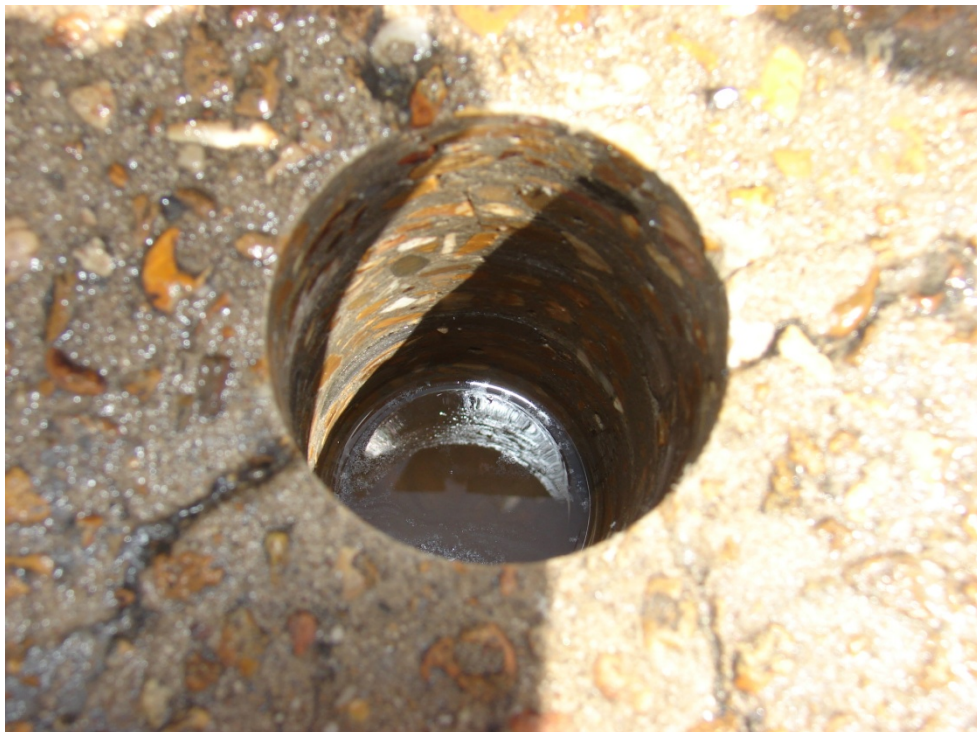
Figure 3 Cracked deck in span 99 northbound (Note the crack depth here was about 2.5 inches)
