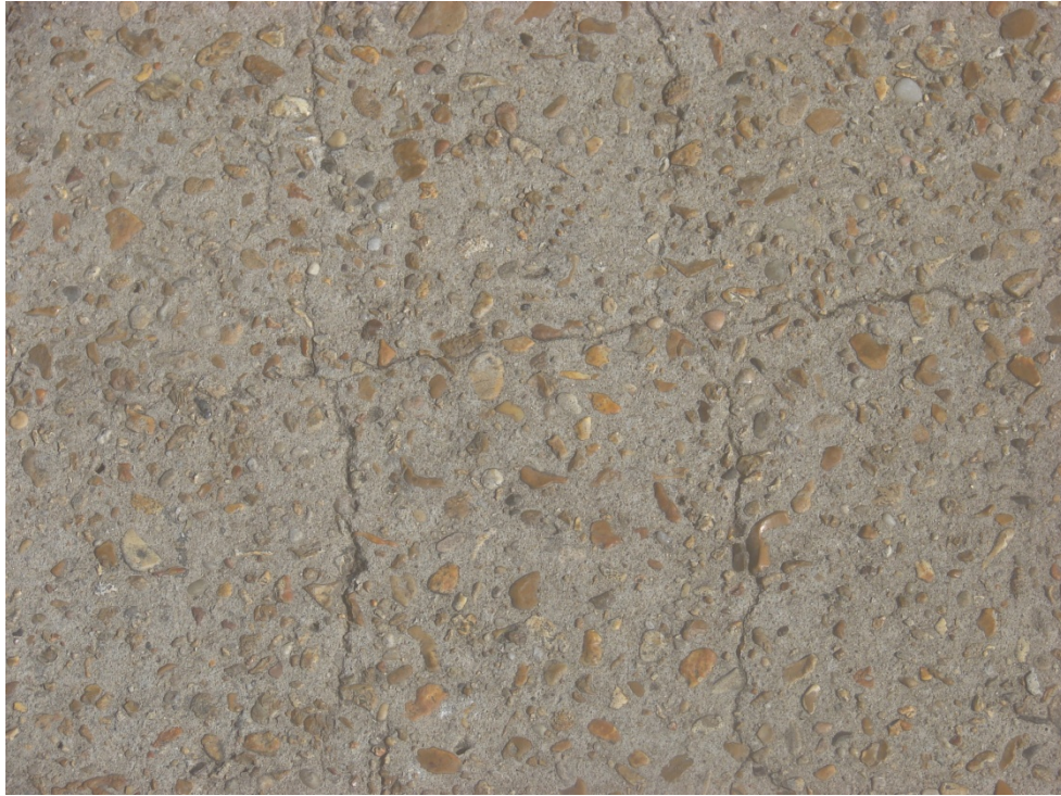
Figure 2 Exposed aggregate and crack pattern (Note the crack pattern is approximately 4 – 6 inches square)
