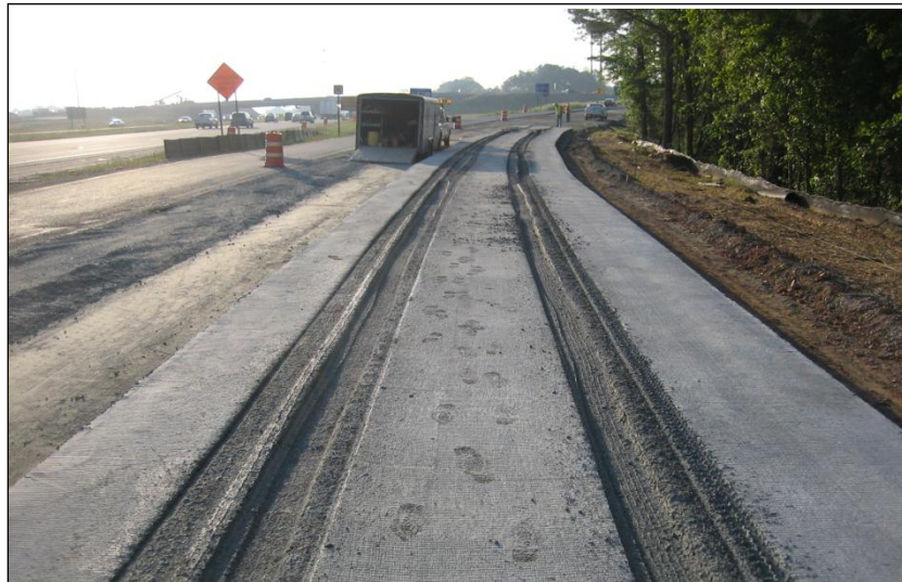
Figure 5.12 Damaged concrete pavement
