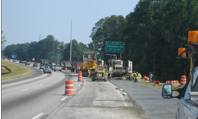
Figure 5.10 Work area issues in Phase 1
