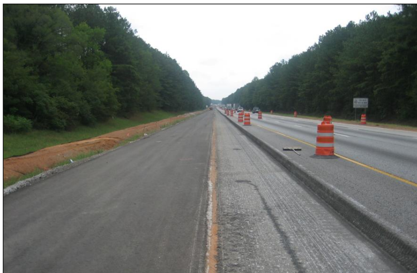
Figure 5.13 Insufficient asphalt base under travel lanes
