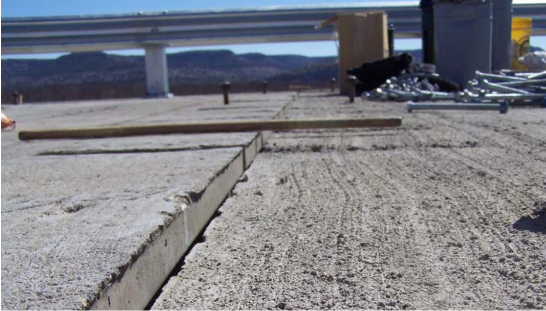
Figure 2: A wooden stick placed at the intersection of two full depth precast panels that have been adjusted using grade bolts. The difference in panel height is over \frac{1}{4} ".
