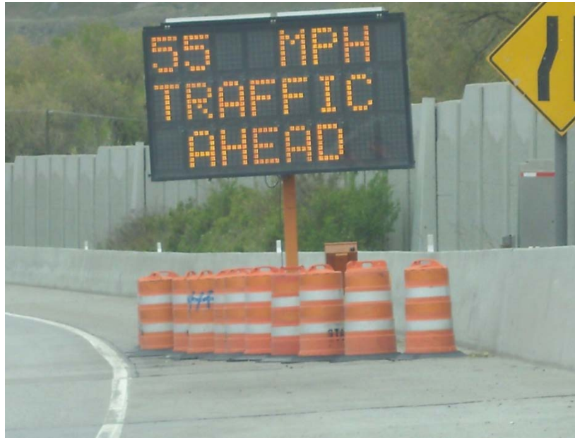
Figure 3-8 VMS 2 final location (taken by Aaron Wilson).
