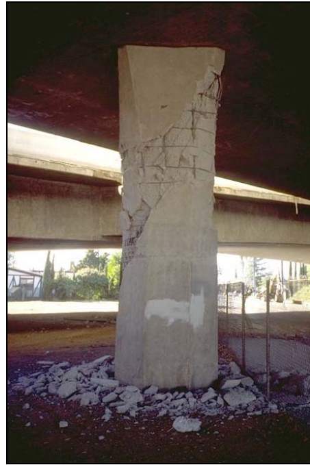
Figure 40. Severe Damage: Brittle shear failure (NISEE)
