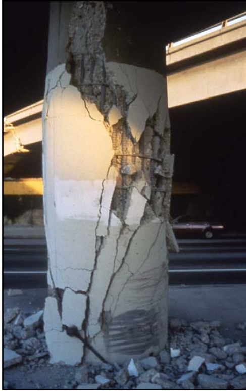
Figure 60. Earthquake damage to reinforced concrete bridge column (Aboutaha)
