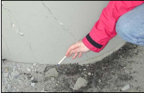
Figure 32. Ground movement indicating possible foundation problem (MCEER)
