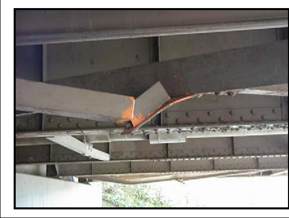
Figure 25. Moderate Damage: Fracture of lower lateral bracing (MCEER)
