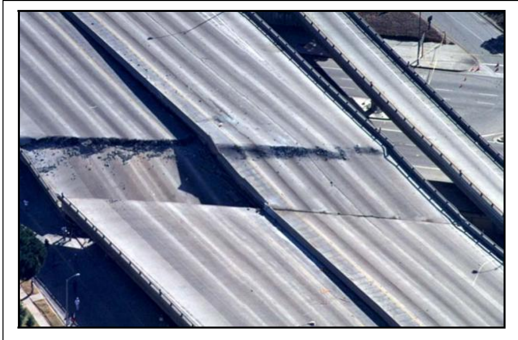
Figure 31. Severe Damage: Deck collapse (USDOT) (I-10 and SR 118 Damage from Northridge EQ http://itsdocs.fhwa.dot.gov/jpodocs/repts_te/13775.html )
