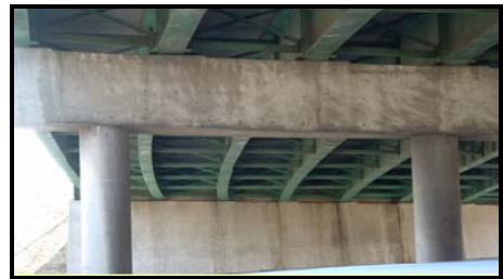
Figure 8c. PBDA Column #3 Substructure Damage
