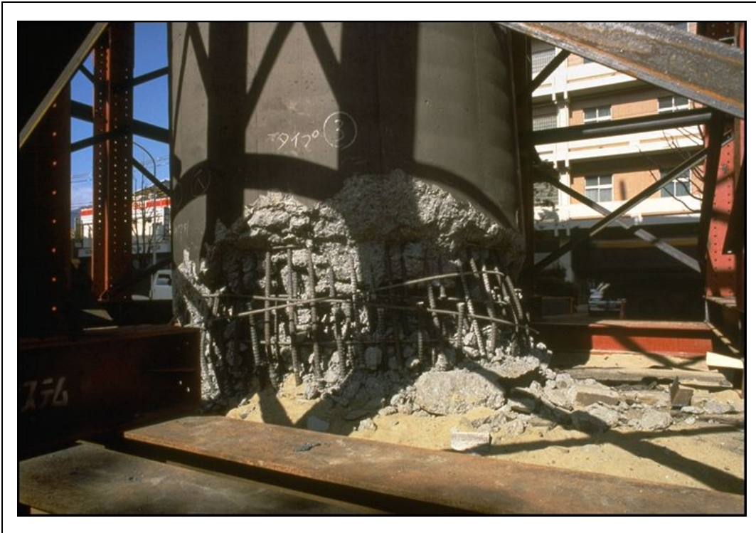
Figure 41. Severe Damage: Weld failure of column longitudinal reinforcement (MCEER)
