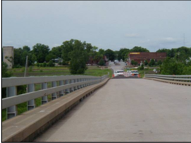
Figure 55. Moderate Damage: Bowing of parapet and railing (MO)
