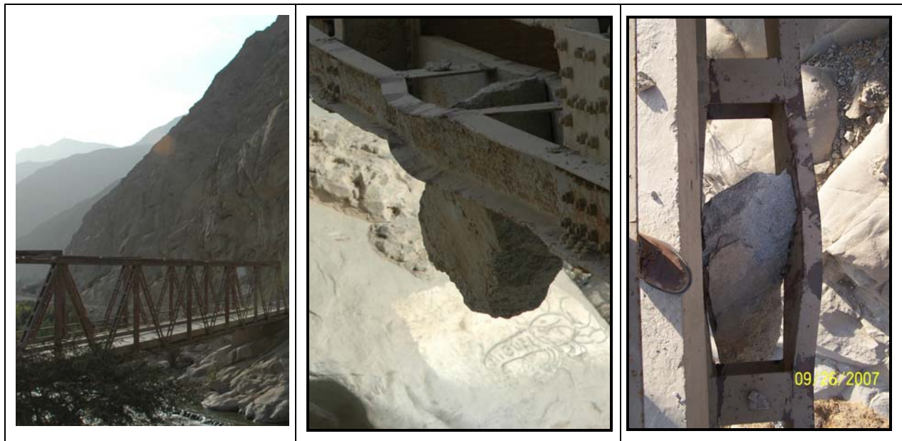
Figure 1. Damage from Rockfall in Peru. (O'Connor)
