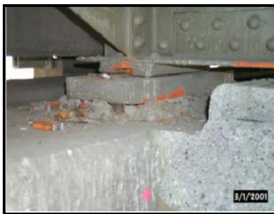
Figure 8d. PBDA Column #4 Bearing Damage
