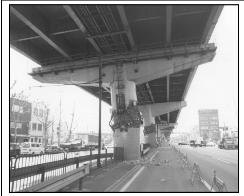
Figure 36. Severe Damage: Mid-height flexural damage (PEQIT)
