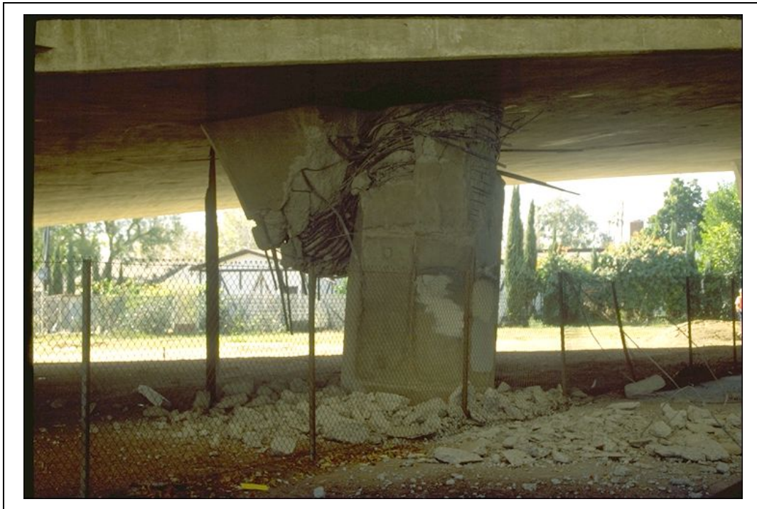
Figure 42. Severe Damage: Shear failure (1971 San Fernando Earthquake) (MCEER)
