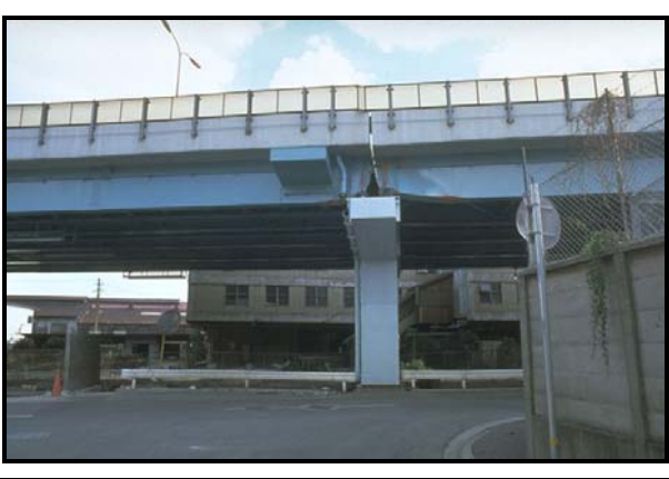
Figure 26. Severe Damage: Steel girder buckling (MCEER)
