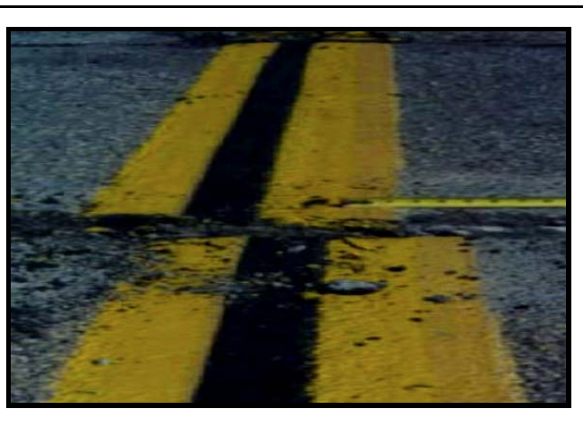
Figure 44: Minor Damage: Transverse movement along the centerline (COHMR)
