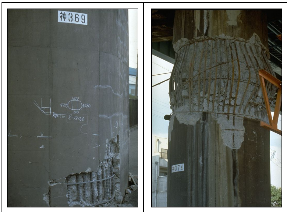
Figure 37. Moderate to Severe Damage: Spalled column; buckling of primary reinforcement (MCEER)
