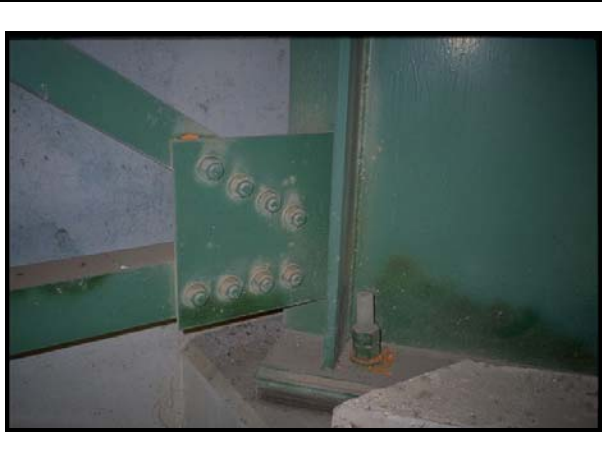
Figure 24. Minor Damage: Damage to anchor bolts (MCEER)
