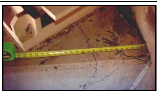
Figure 47. Minor Damage – Cracks induced by steel bearing (CPHMR)
