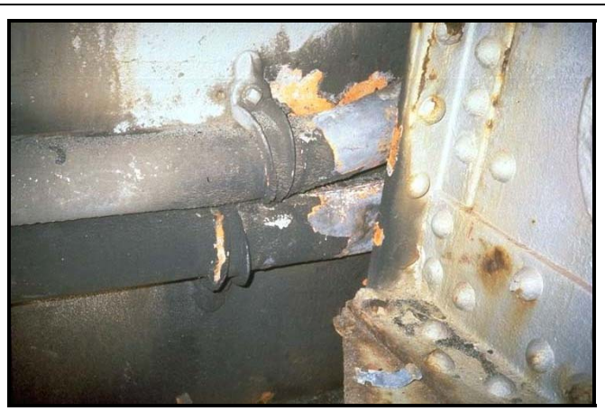
Figure 57. Movement of Trusses at Pier 23 of the San Francisco Oakland Bay Bridge during the Loma Prieta Earthquake. The shoe (at the right) hit two pipes that carried electric wires and dented them. These dents indicated that there was at least 3 to 4 inches of movement. (NISEE)
