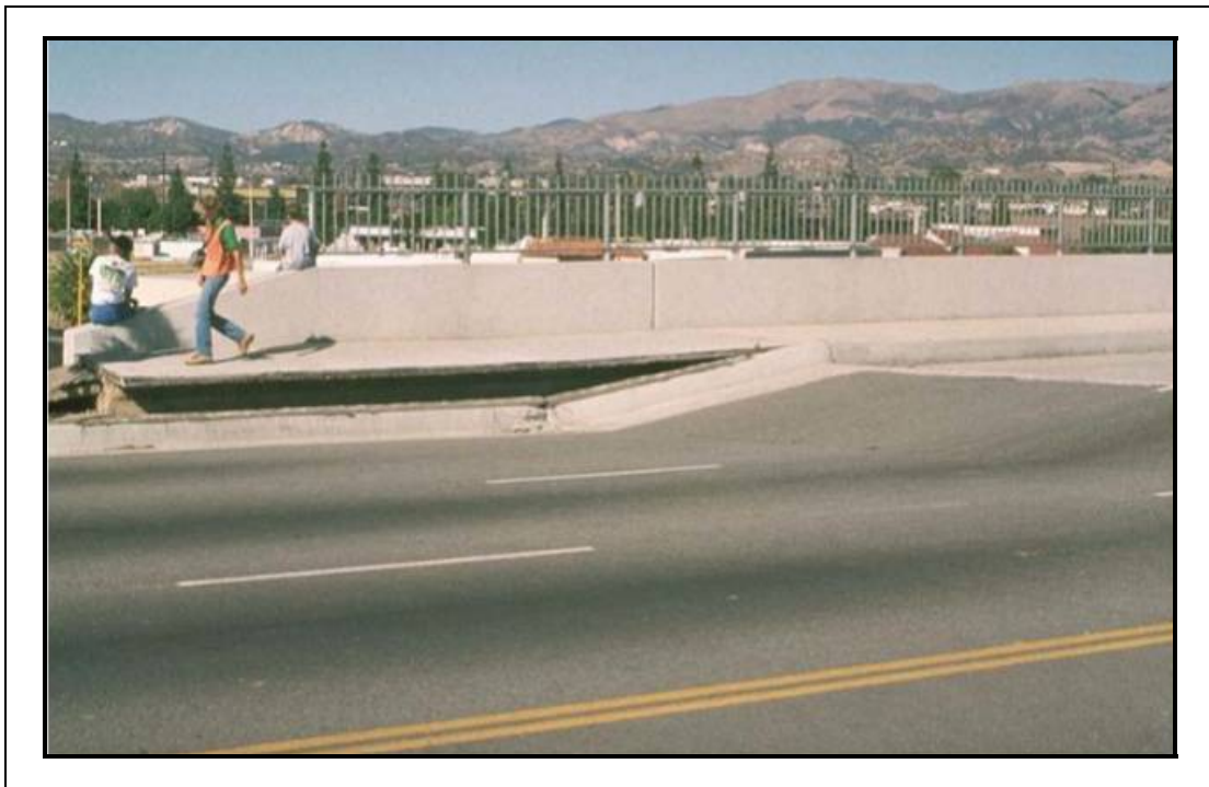
Figure 16. Settlement of bridge approach, considered Major damage (KTC)
