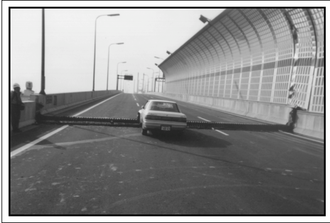
Figure 45: Moderate Damage: Differential settlement and expansion joint damage (PEQIT)
