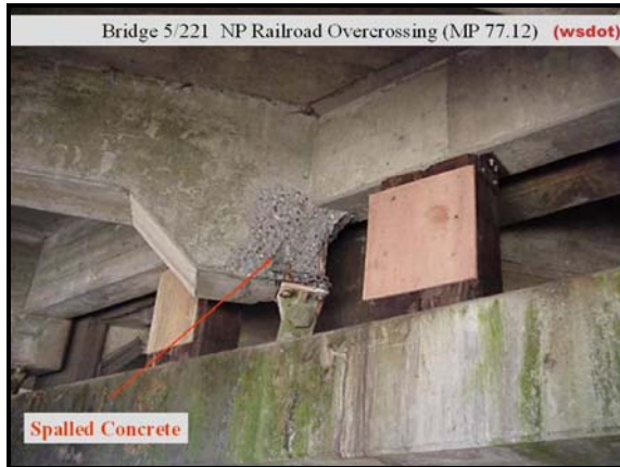
Figure 19. Moderate Damage: Spalled concrete (WSDOT)
