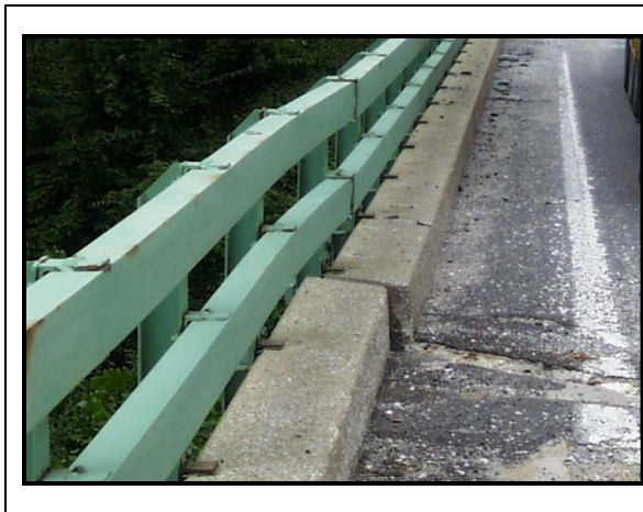
Figure 56. Misalignment of curb line and bowing of railing. Notice that the white edge line is slightly shifted at the joint. (MO)
