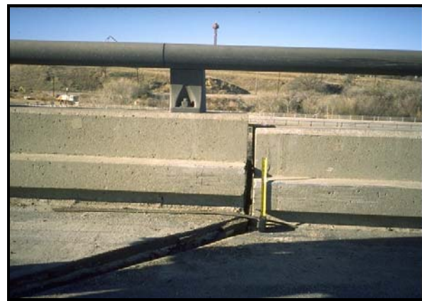
Figure 28. Minor to Moderate Damage: Vertical and horizontal movement at joint (NISEE)
