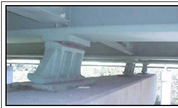
Figure 46. No Damage: Tilted rocker bearings, movement due to thermal loads (INDOT)
