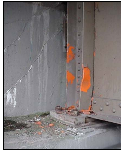
Figure 22. Minor Damage: Web stiffener damage. Note that the paint has flaked off recently. (MCEER)
