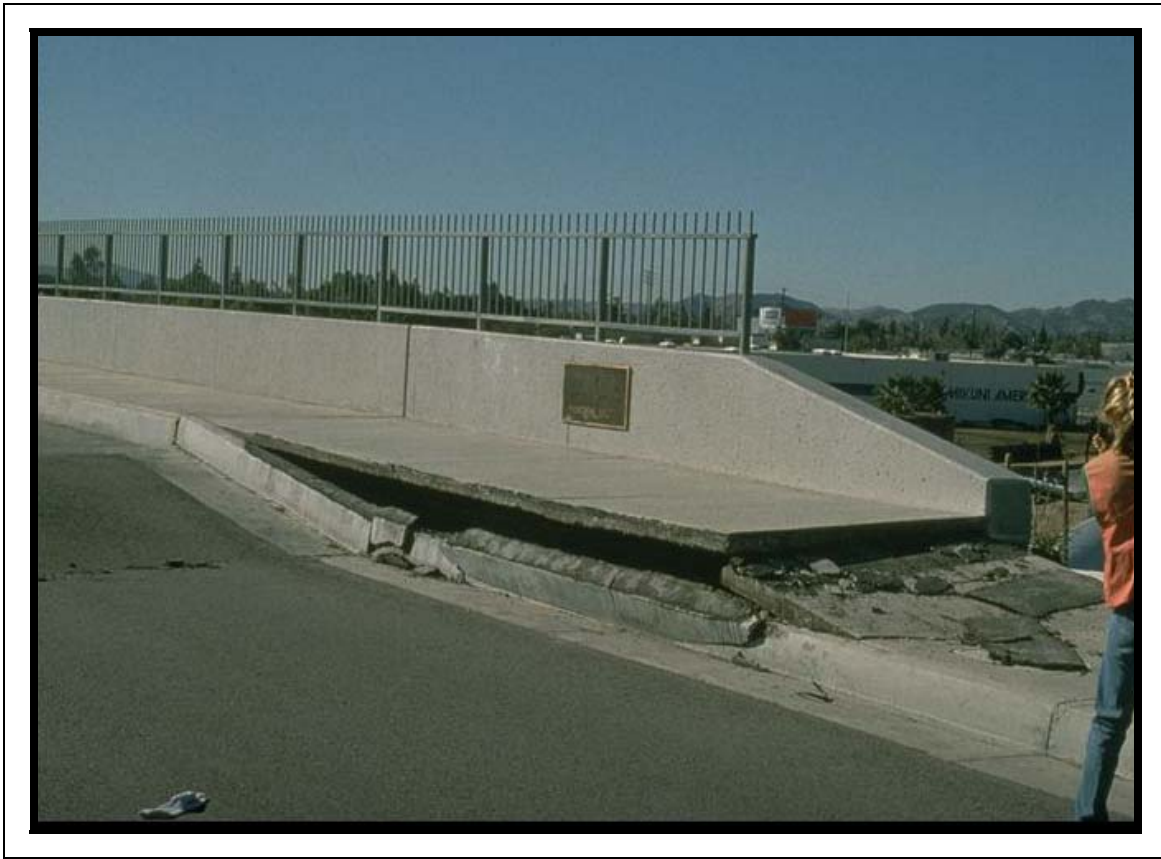
Figure 18. Settlement at the bridge approach, likely caused by soil settlement around the abutment (Northridge EQ) (NISEE)
