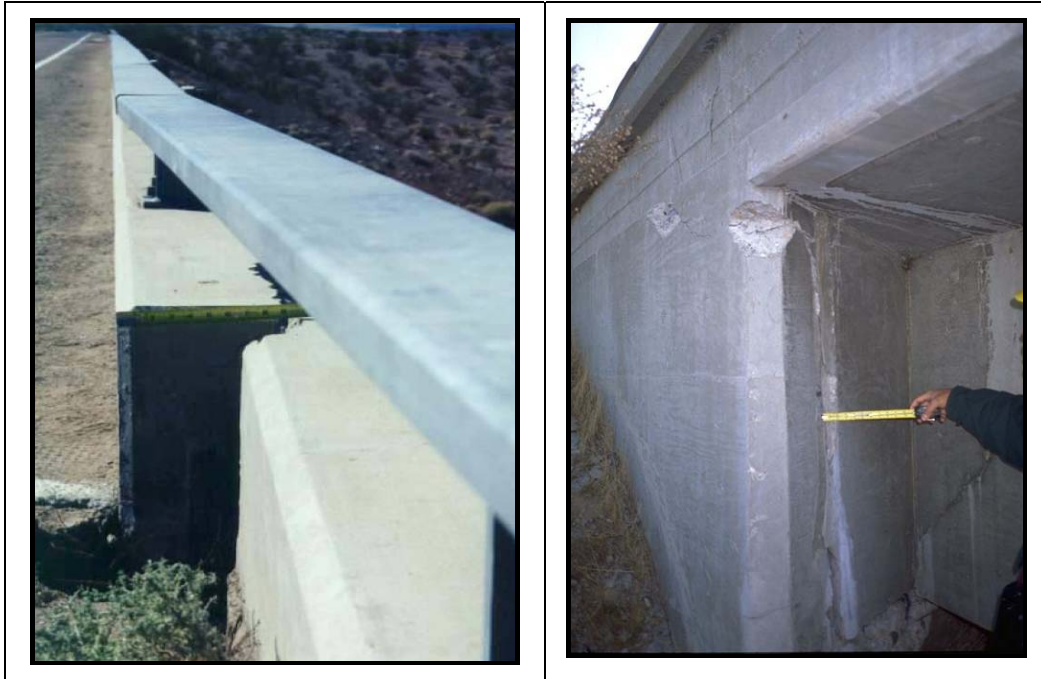
Figure 58. Moderate Damage: Transverse movement of the abutment wing-wall (CPHMR)
