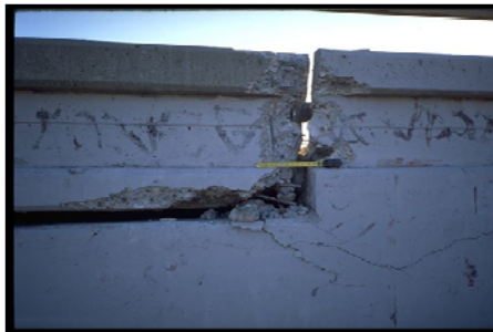
Figure 11. Evidence of Longitudinal Pounding (NISEE)
