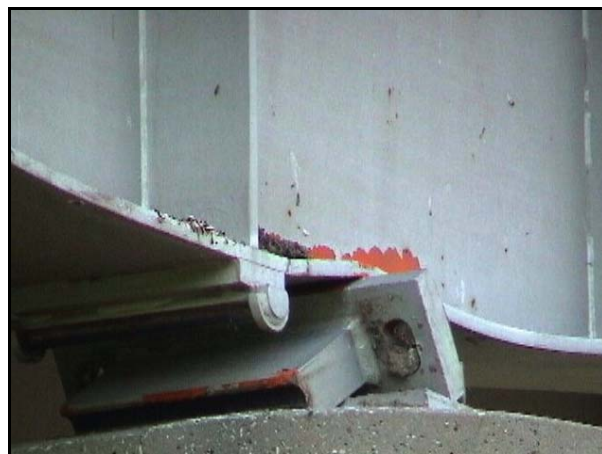
Figure 49. Severe Damage: Toppled rocker bearing (MO)
