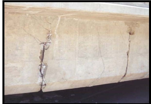
Figure 20. Moderate Damage: Flexural cracking of concrete girder (KTC)
