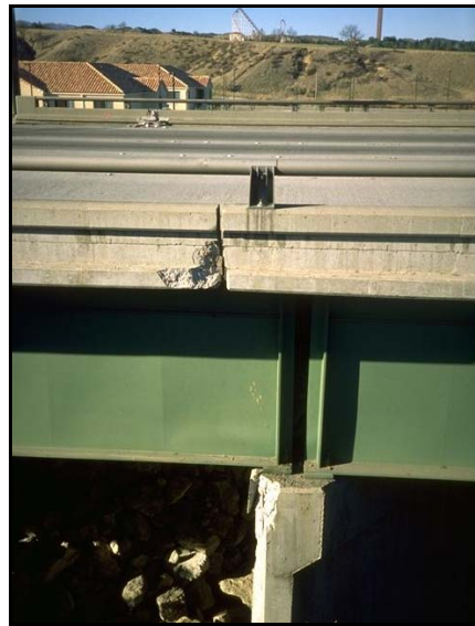
Figure 35. Moderate Damage: Support damage at top of pier. Minor Damage: Fascia concrete (MCEER)
