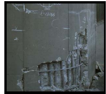
Figure 12. Spalling and Splice Failures at Column Base (NISEE)
