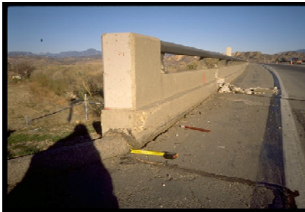
Figure 10. Settlement at Approach: Spalling (NISEE)
