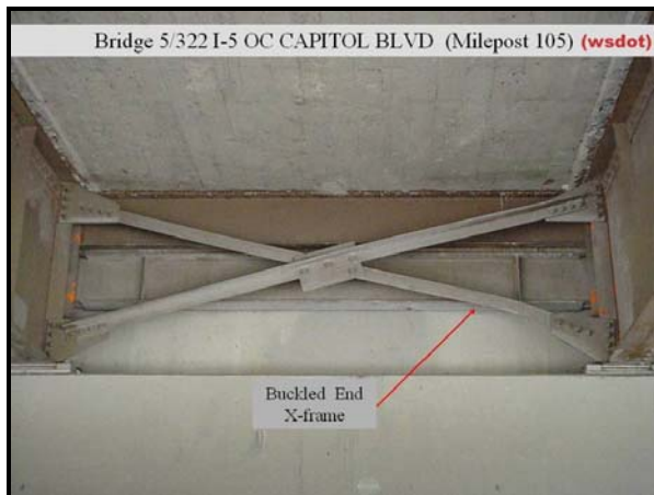
Figure 21. Minor Damage: Buckled bracing element. (WSDOT)
