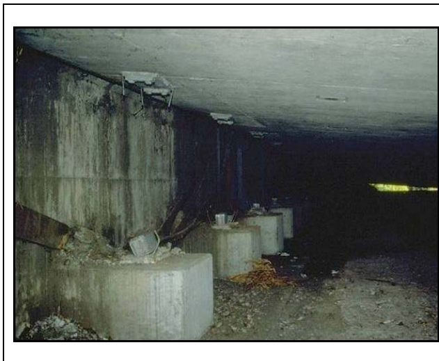
Figure 48. Moderate Damage: Abutment rocker bearings. (MCEE)
