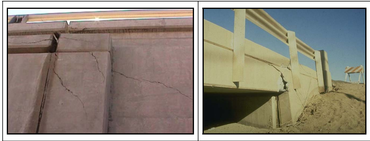
Figure 52. Minor Damage: Shear cracking at the abutment wing-wall (KTC)
