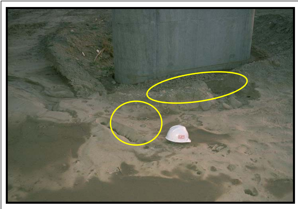
Figure 17. Evidence of liquefaction near a pier (NISEE)
