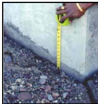
Figure 8e. PBDA Column #5 Soil Problems
