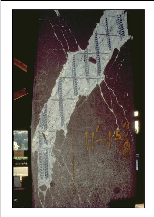
Figure 39. Moderate Damage: Column shear (NISEE)
