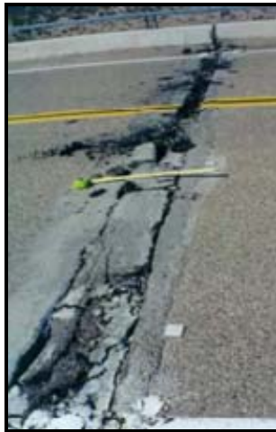
Figure 8b. PBDA Column #2: Superstructure Damage
