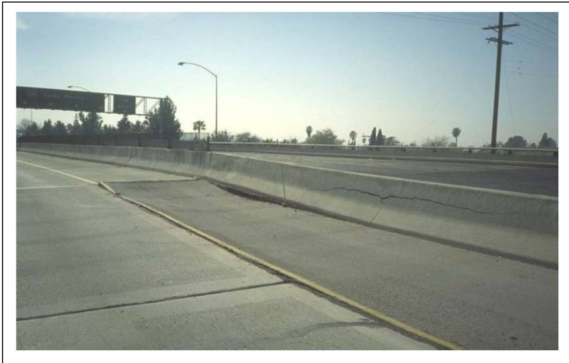
Figure 14. Moderate Damage: Approach slab settlement (Sardo, A. G., et al., 2006). Note the cracking of the concrete barrier as well.
