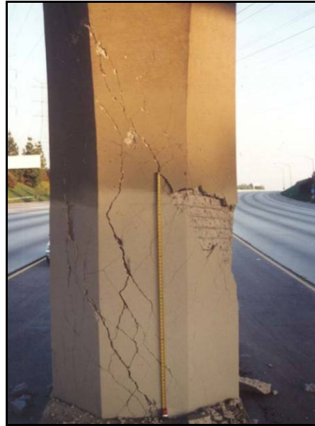
Figure 33. Minor Damage: Cracking and spalling of the concrete cover at the column base (KTC)
