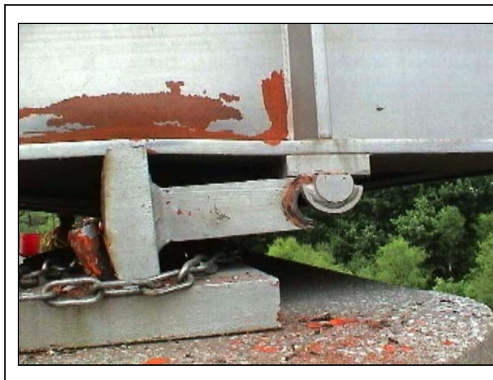
Figure 50. Severe Damage: Rocker bearing failure (MO)
