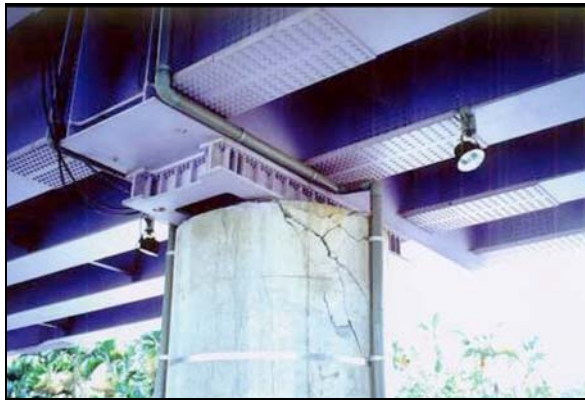
Figure 34. Moderate Damage: Compression failure at top of concrete column (INDOT)
