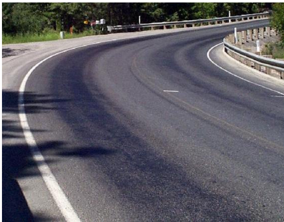
Figure 1. Flushing HMA on SR 20 soon after placement.
