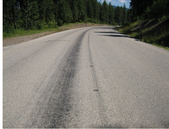
Figure 4. Test Section 1 (on left) with 0.27 gal/sy shows flushing in the wheel path soon after construction while no flushing was present in Test Section 3 (on right) at 0.20 gal/sy.
