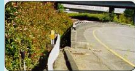
Before: Outdated guardrail at the SR 7/SR 705 interchange with I-5 in Tacoma.
