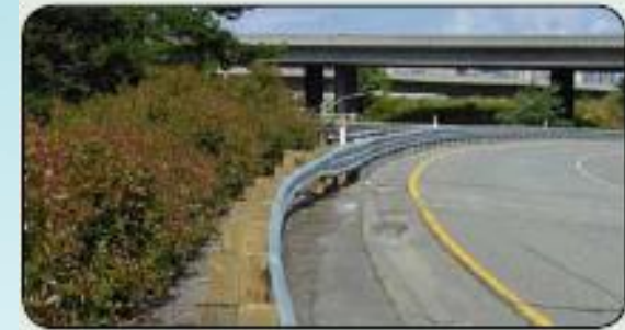
After: The replacement guardrail meets current safety standards, and creates a continuous transition to the bridge rail, removing the blunt end that had existed previously.
