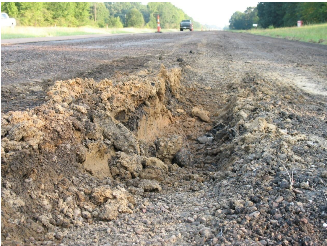
Figure 14: Surface Deformation Due to Subgrade Pumping
