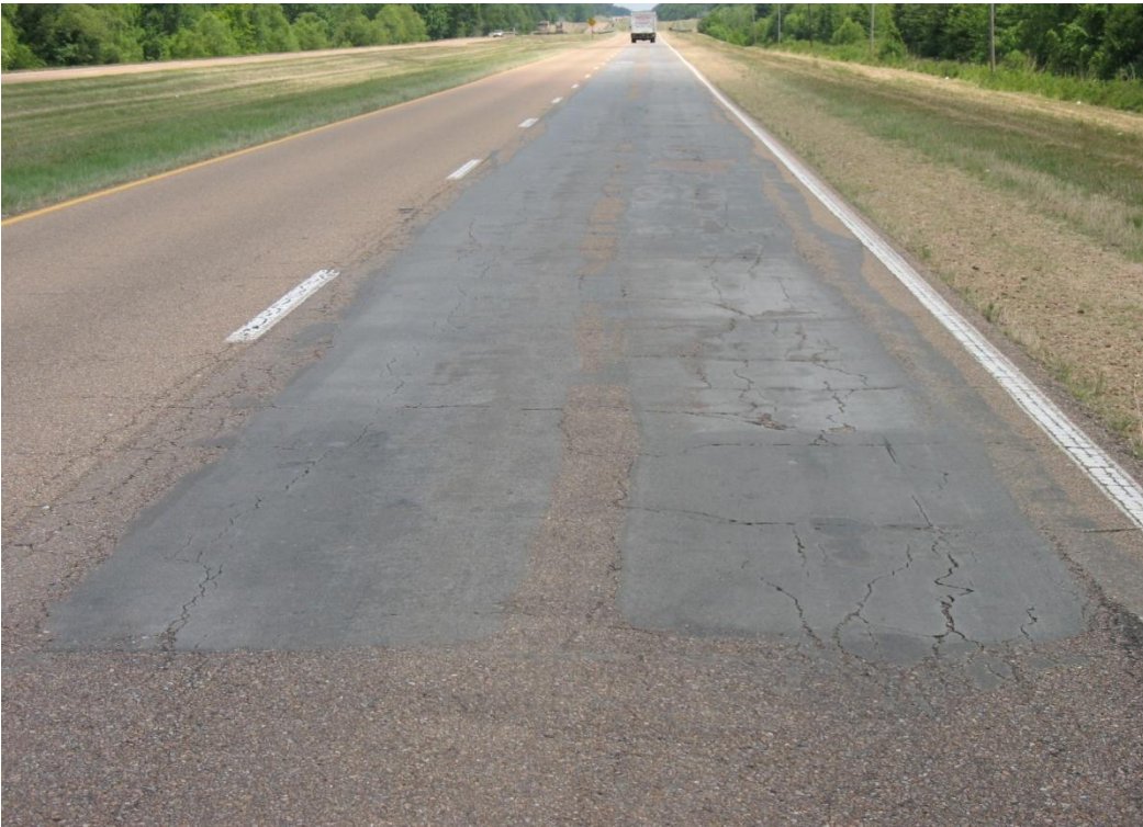
Figure 4: Rutting, Compound/Longitudinal Cracking
