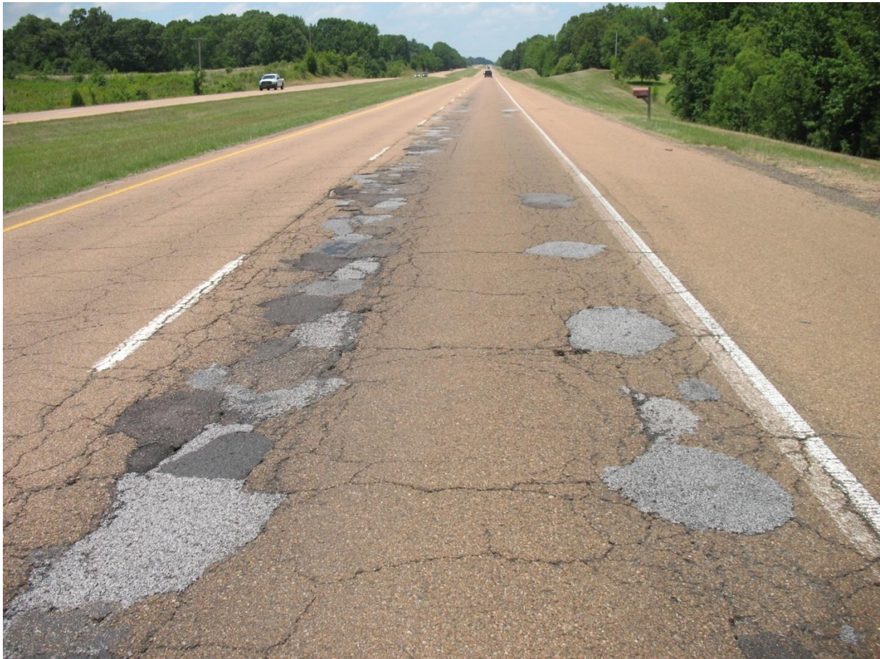
Figure 2: Pothole Repair and Wheelpath Deterioration
