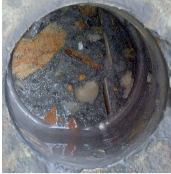
Figure 56. Structure 2866, Bent 67, Pile H, Exposed Reinforcement
