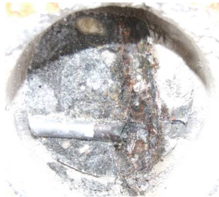
Figure 61. Structure 2900, Bent 45, Pile B, Exposed Vertical Strand
