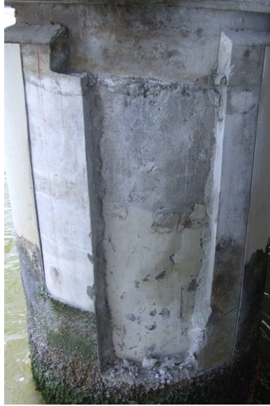
Figure 20. Mortar Without Reinforcement
