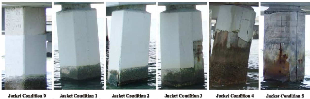
Figure 10. Visual Condition Rating of Fiberglass. Condition ratings are described in Table 2.
