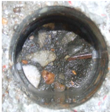
Figure 64. Structure 2902, Bent 23, Pile C, Exposed Reinforcement
