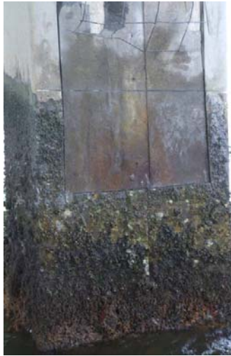
Figure 53. Saturated Mortar Behind Fiberglass
