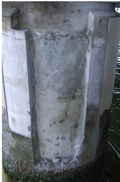
Figure 57. Structure 2900, Bent 45, Pile A, Improper Reinforcement
