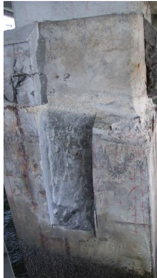
Figure 63. Structure 2902, Bent 23, Pile C, Exposed Substrate
