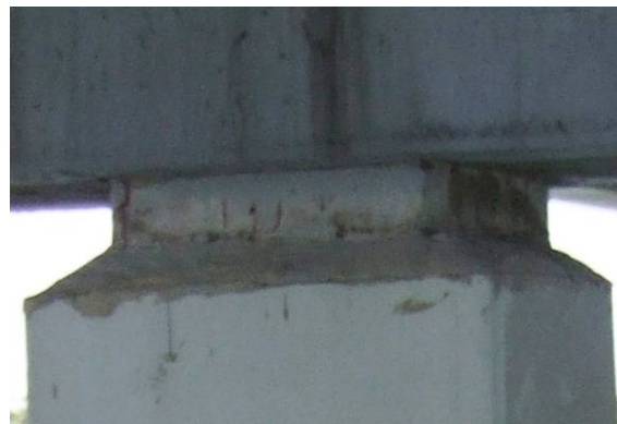
Figure 9. Substrate Exposed Above Jacket
