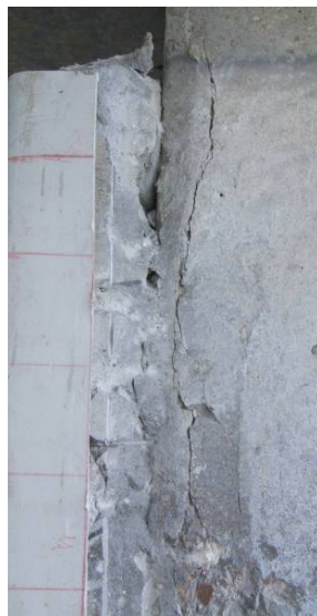
Figure 54. Structure 2866, Bent 67, Pile G, Vertical Crack in Substrate Beneath Mortar
