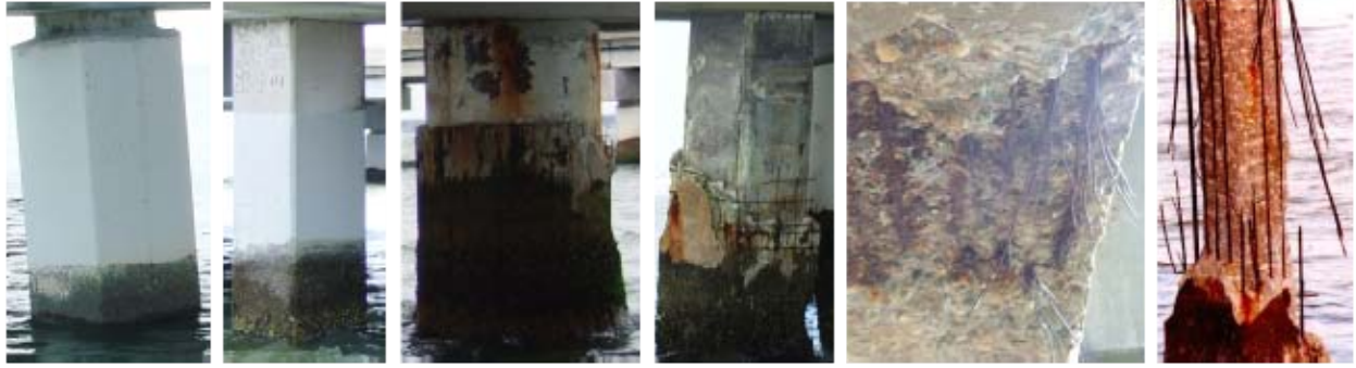
Figure 12. Visual Condition Rating of Substrate. The ratings are described in Table 2. The photograph for Condition 4 (*) is from the Route 615 Chickahominy River Bridge in Virginia, not HRBT. The photograph for Condition 5 (**) is from the St. George Island Bridge in Florida, not HRBT ( Source: Hartt and Rappa, 1998 ). Conditions 4 and 5 were not observed on HRBT during this study.
