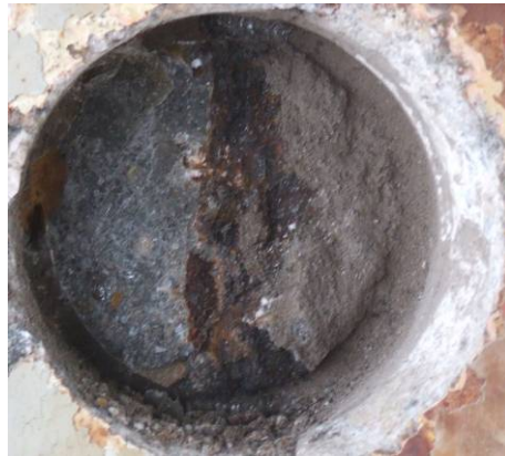
Figure 65. Structure 2900, Bent 5, Pile B, Exposed Vertical Tendon
