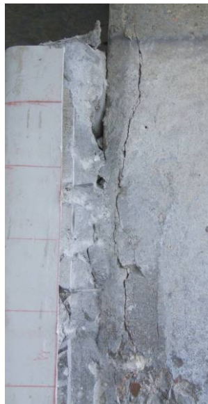
Figure 21. Vertical Crack Beneath Mortar
