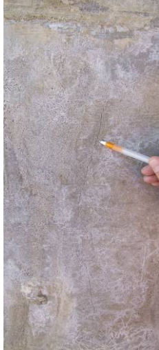
Figure 58. Structure 2900 Bent 45 Pile A, Vertical Crack Beneath Mortar
