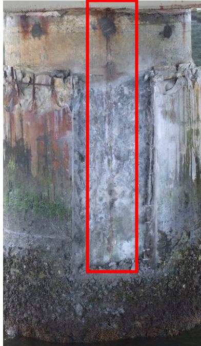
Figure 60. Structure 2900, Bent 45, Pile B, Exposed Substrate
