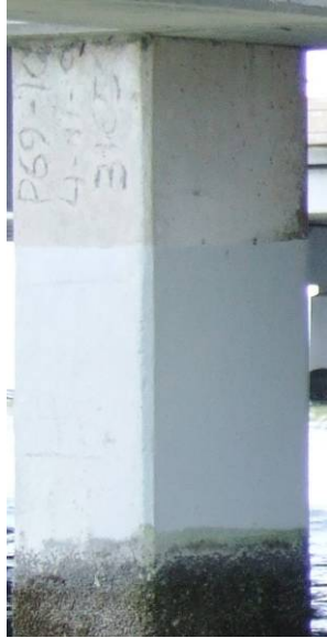
Figure 17. Epoxy-Coated, Not Jacketed, Pile
