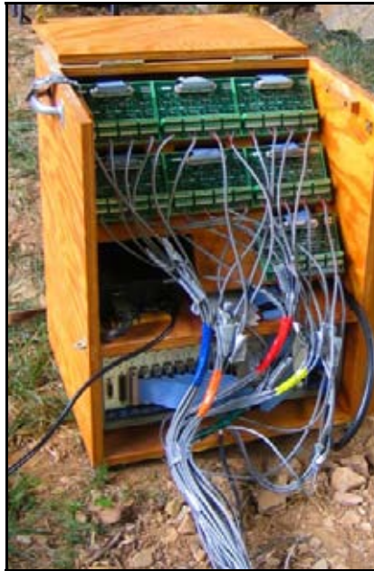
Figure 9. Connection to Data Acquisition System
