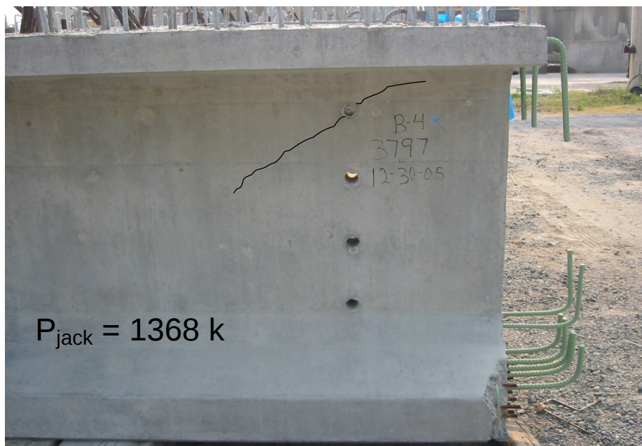
Figure 16. PCBT-53 Anchorage Zone Case Study – Fair Condition
