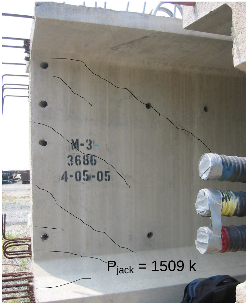
Figure 18. PCBT-77 Anchorage Zone Case Study – Poor Condition
