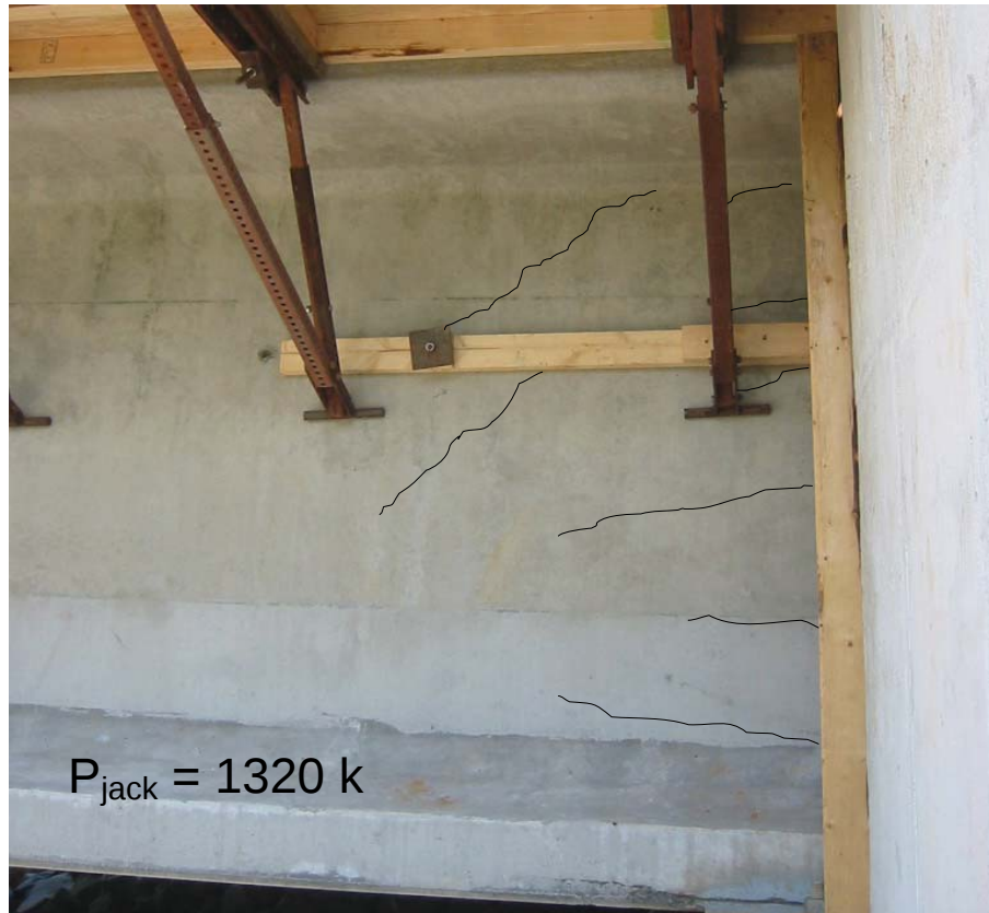
Figure 19. PCBT-77 Anchorage Zone – Poor Condition
