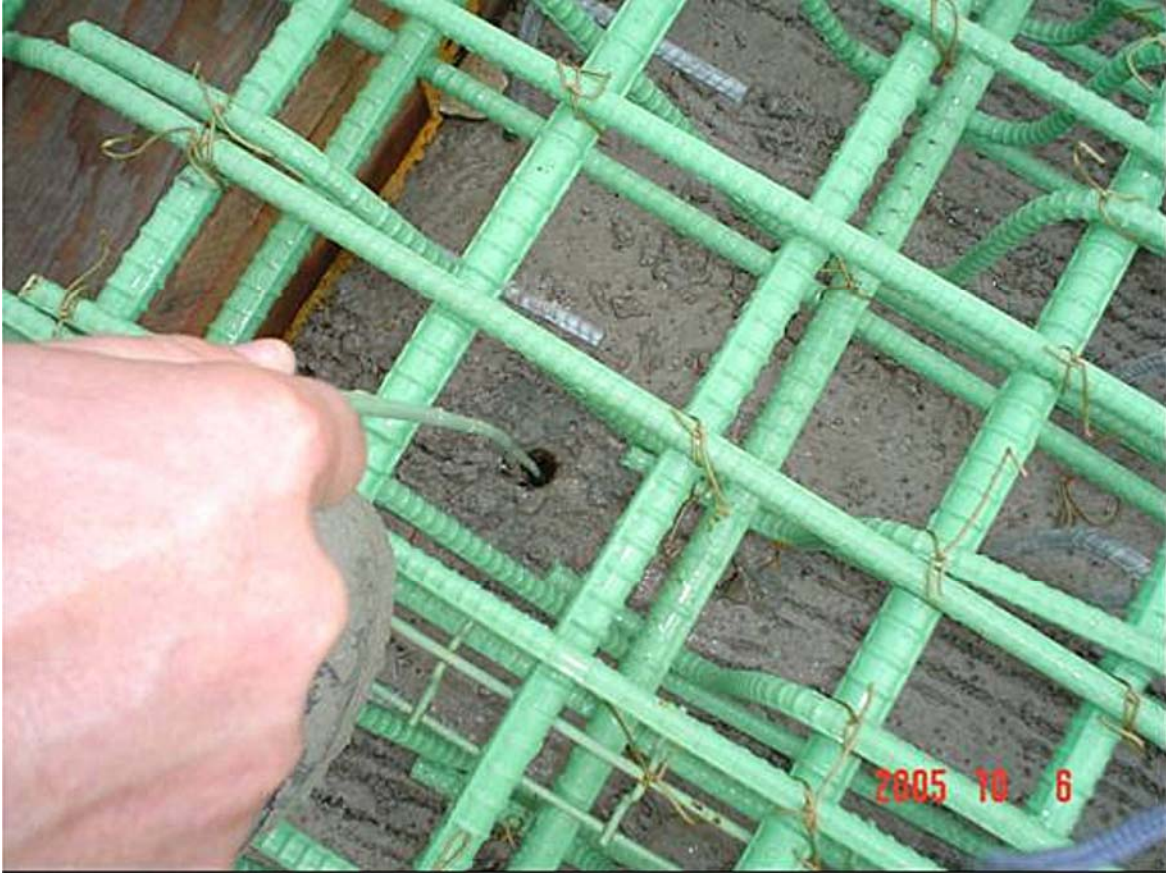
Figure 13. Example of ECR Showing Wire Ties and Bar Surfaces
