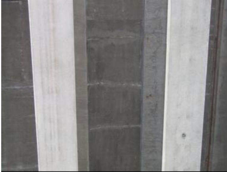
Figure 27. Efflorescence Pattern Between Two Girders on Underside of Northbound (MMFX 2) Deck With Joint for Northbound/Southbound Decks Visible at Right
