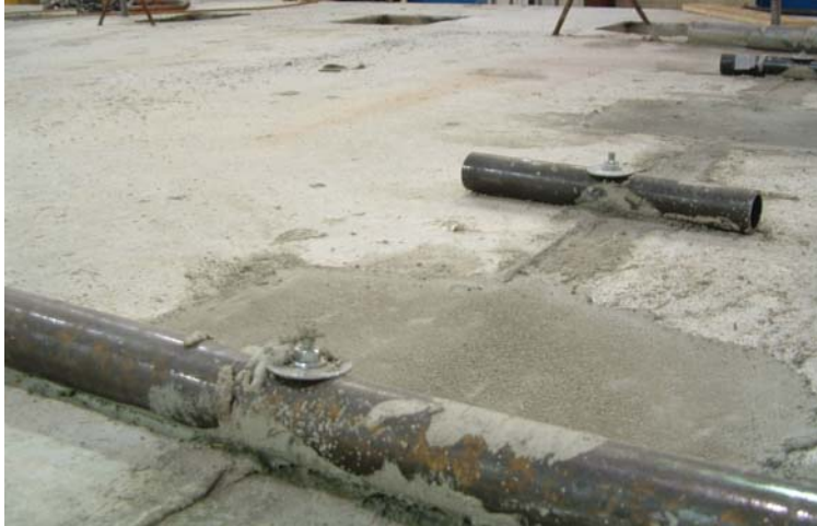
Figure 24. Grouted Female-Female Joints with Steel Pipe and Threaded Metal Rod Forming Alternative.
