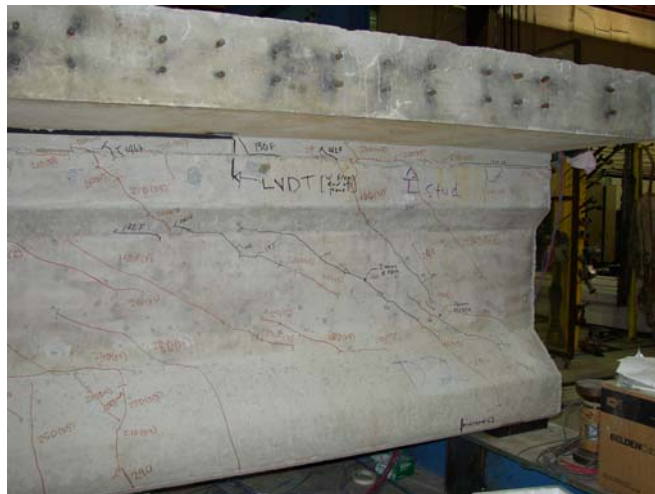
Figure 44. Cracking Pattern at Dead End for Girder 2 During Final Static Test.
