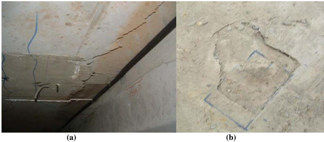
Figure 40. Punching Shear Failure at Dead End (a) Bottom Surface of Deck (b) Top Surface of Deck.
