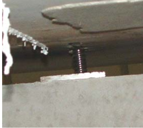
Figure 23. Leveling Bolt Bearing on Steel Plate.
