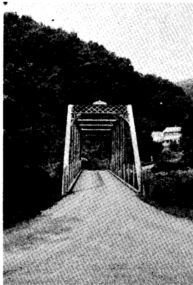
Figure 8. King Iron Bridge & Manufacturing Co. Pratt truss, with bridge plate intact, built in 1892. (Montgomery Co., photo #12455-9)
