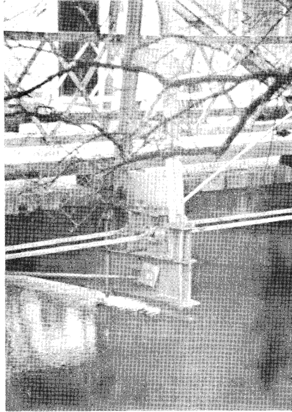
Figure 4. A pin connection used at the junction of an intermediate post, a lower chord member, a diagonal and a hanger beam. (King William County; see form/photo number 06-50-1.)
