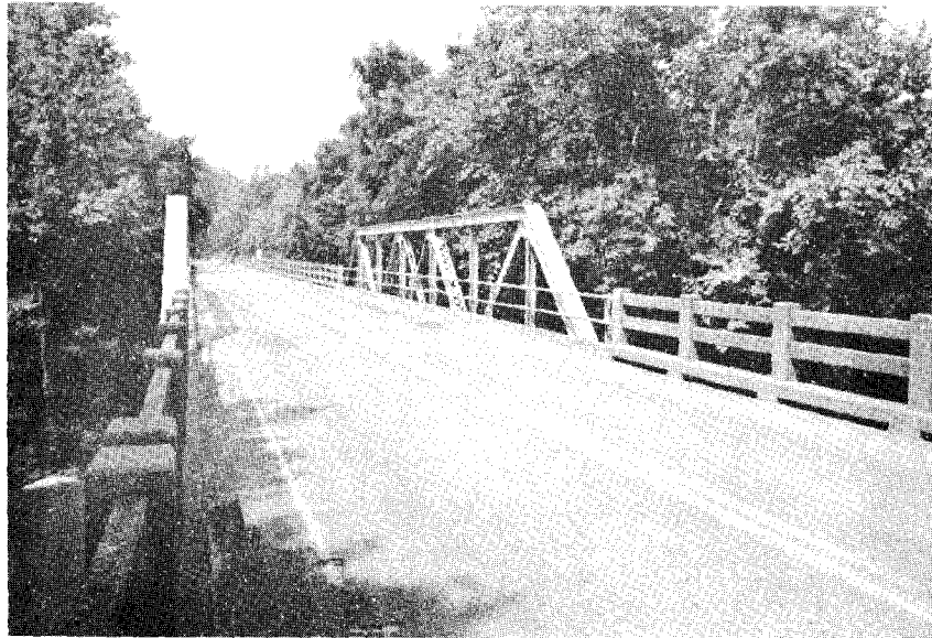
Figure 4. Five-span, two-lane bridge with a 90-foot low/pony triangular truss built by Bethlehem Fabricators, Inc., Bethlehem, Pennsylvania, according to plans and specifications prepared by the Virginia State Highway Commission in 1927. (Fairfax/Prince William County line; see form/photo number 07-76-1.)
