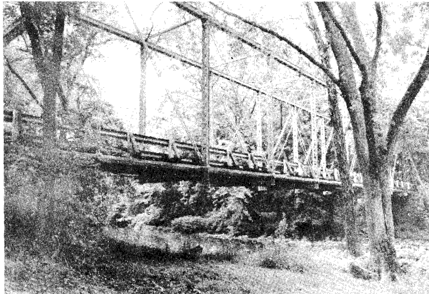
Figure 14. Single-span, through/high Pratt truss of unusual length built by the Variety Iron Works Company, Cleveland, Ohio; date unknown. (Loudoun County, see form/photo number 07-53-6.)
