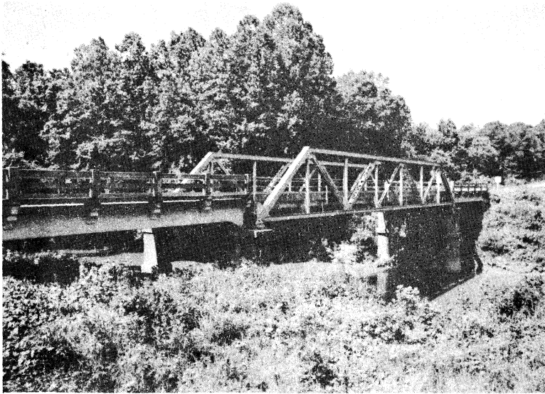
Figure 6. Three-span, two-lane bridge with a 105-foot low/pony triangular truss center span designed in 1929 by the Virginia State Highway Commission, Richmond, Virginia. (Brunswick County; see form/photo number 04-12-4.)
