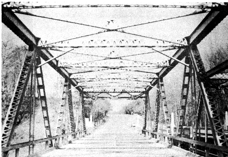
Figure 5. Five-span, two-lane bridge with a 140-foot span through/high triangular truss with horizontal top chords; built in 1926 by the Roanoke Iron & Bridge Works, Inc., Roanoke, Virginia. (Hanover/Caroline County line; see form/photo number 04-42-1.)
