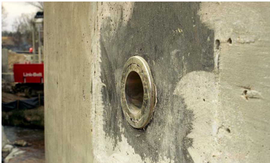
Figure 7. Load Cell at Butress of Abutment B
