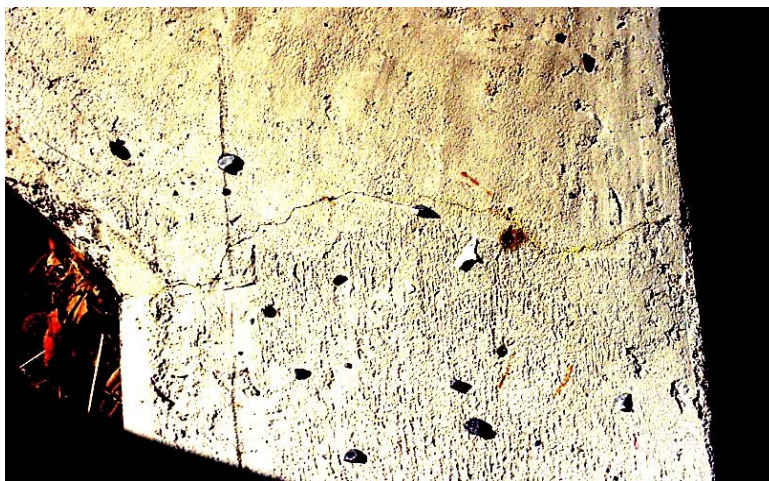
Figure 19. Plan View of Cracked Wingwall at Abutment B
