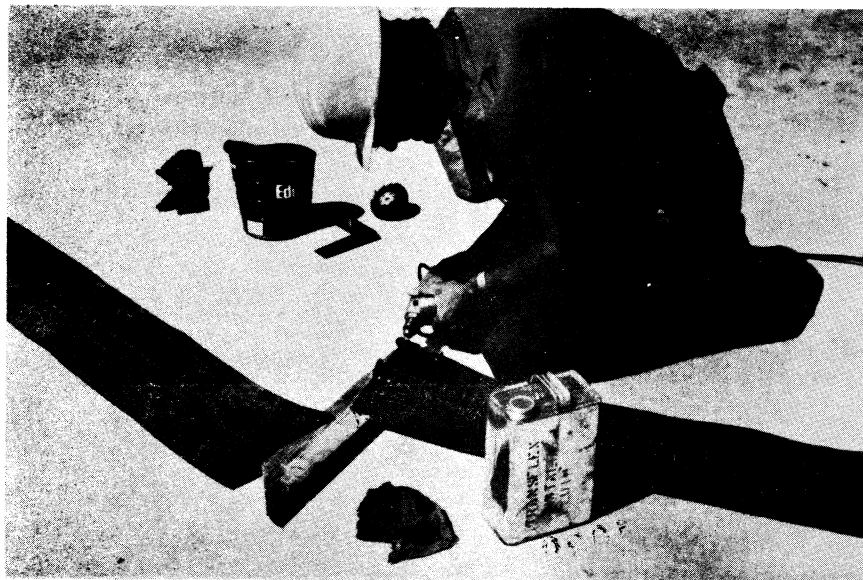
Figure 4. Preparing the surface prior to splicing the two elastomeric membrane sections together.
