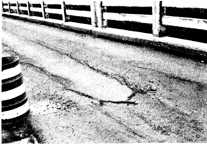
Figure 16. Failure of asphaltic concrete overlay on Witmer membrane.
