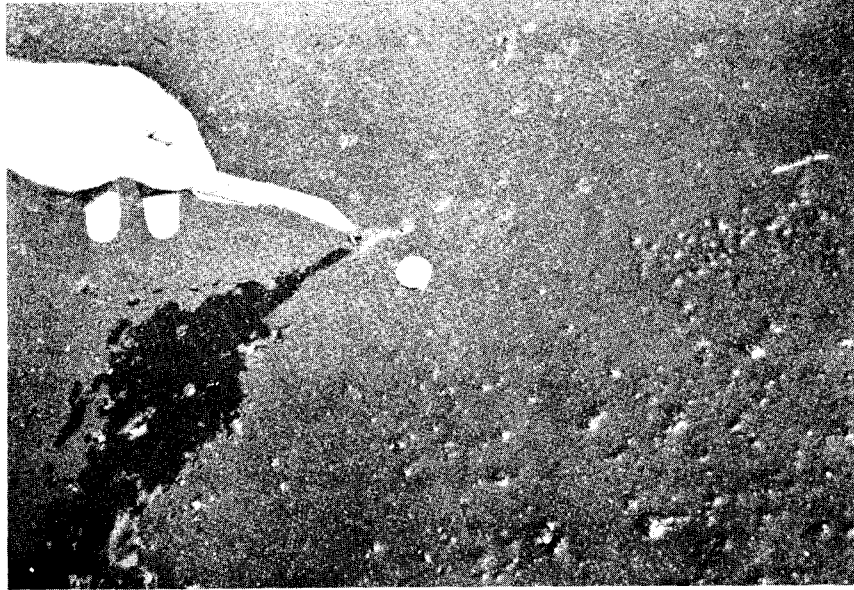
Figure 17. Bubbles in first coat of coal tar epoxy sealcoat.
