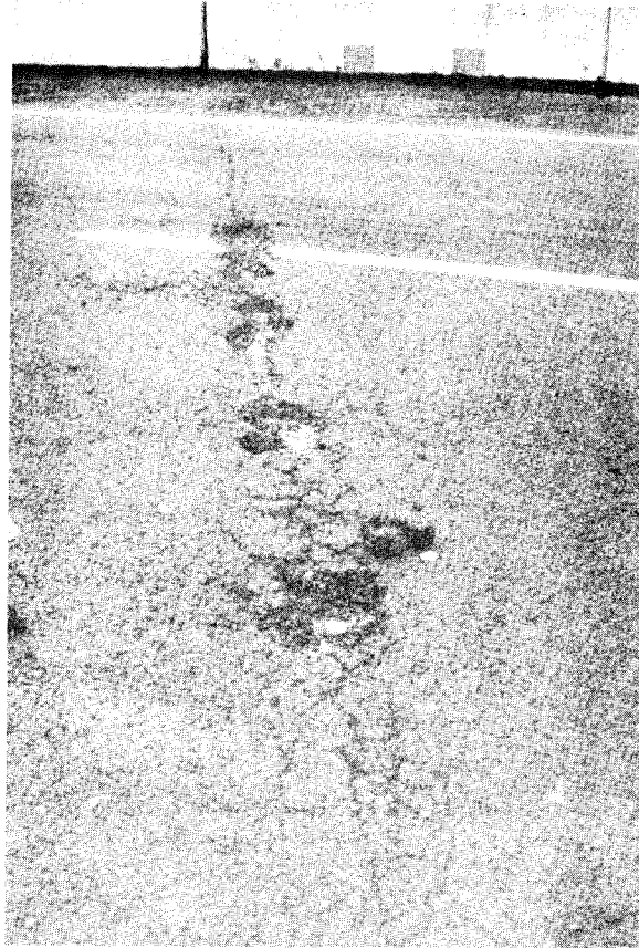
Figure 13. Raveling of asphaltic concrete overlay over deck expansion joints.
