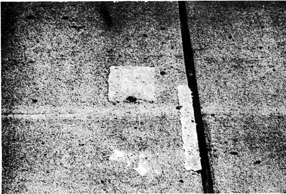
Figure 1. Typical areas requiring patches after slightly more than a year's service. (Guardkote 250 epoxy mortar overlay, SBL Rte. 85 bridge over the Roanoke River.)
