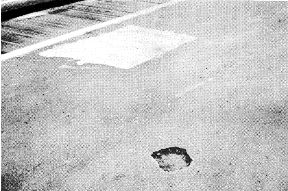
Figure 2. A failure (foreground) which developed three months after the repair shown in the background. (Guardkote 250 epoxy mortar overlay after two years' service, SBL, Rte. 85 bridge over the Roanoke River.)
