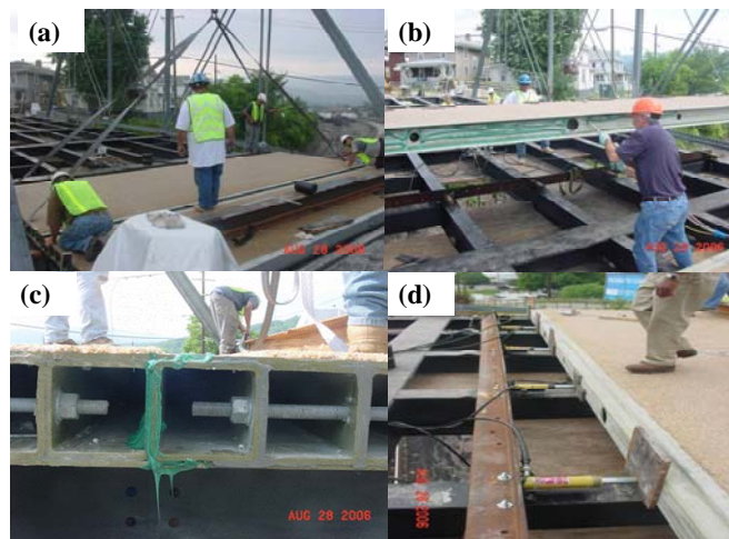
Figure 19. Field installation of the FRP bridge deck (a) Dry fit (b) Adhesive application (c) Seam curing (d) Jacking system
