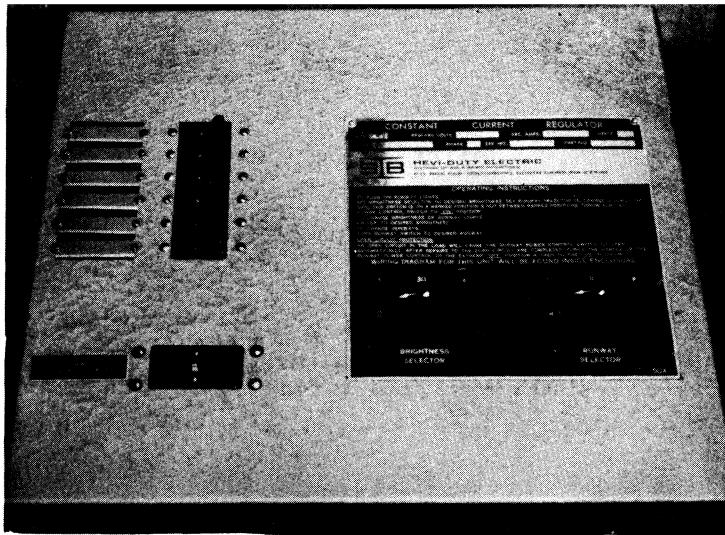
Figure 5. Control panel for constant current regulator.
