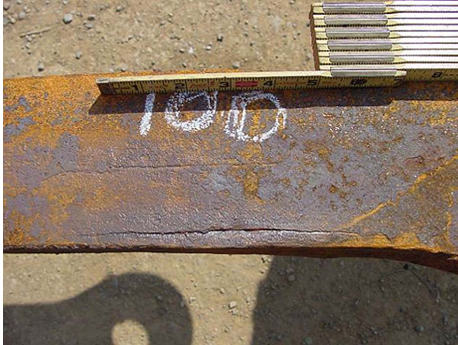
Figure 16. Longitudinal Seams in Face of Lower Chord Eye Bar 100
