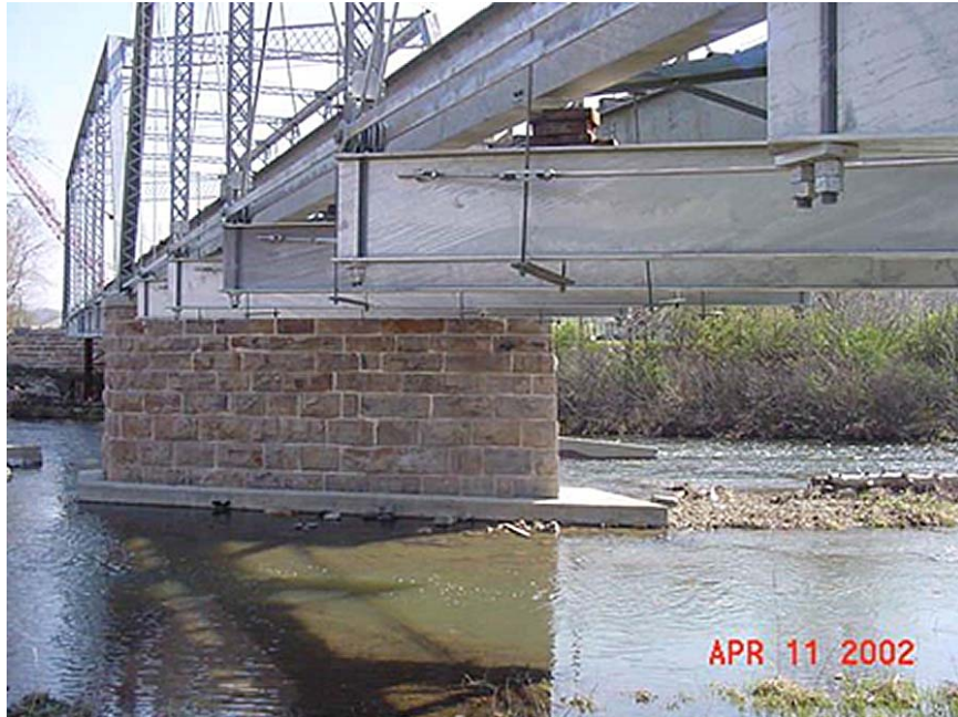
Figure 33. Loosened Falsework Hangers at Completion of Truss Erection
