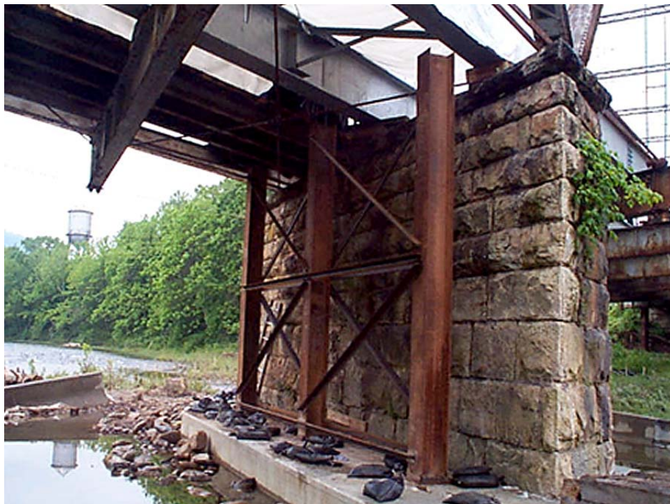
Figure 23. Falsework Bent at Pier with Two Lines of Falsework Beams in Place
