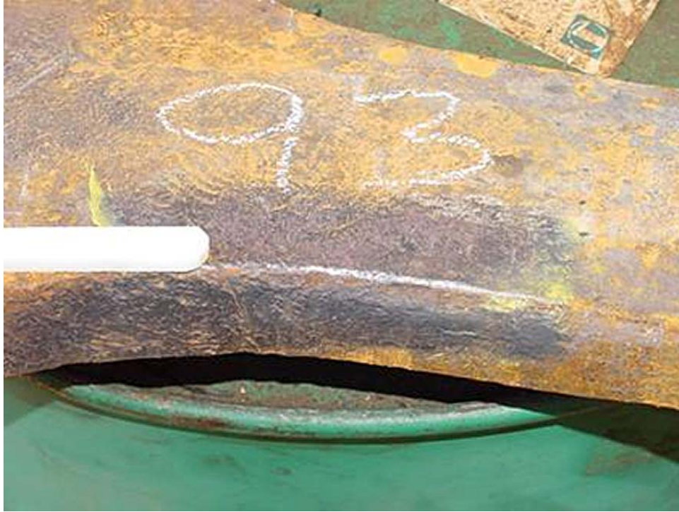
Figure 12. Crack (at Tip of Pointer) in Transition Radial Area on Edge of Bar 93
