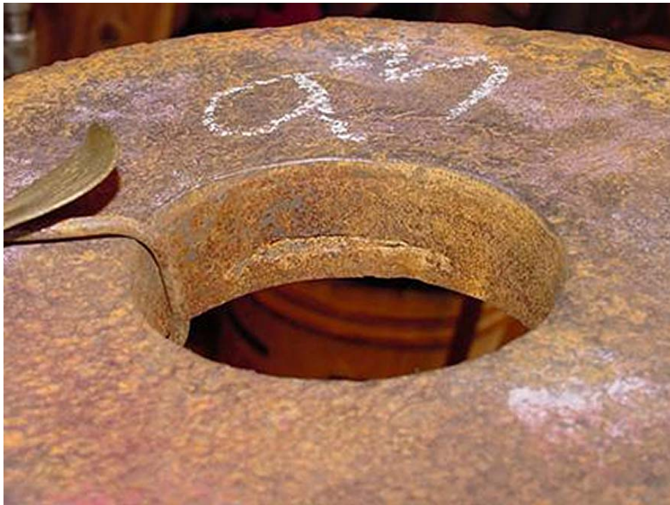
Figure 13. Seam in Surface of Pin Hole, Eye Bar 93
