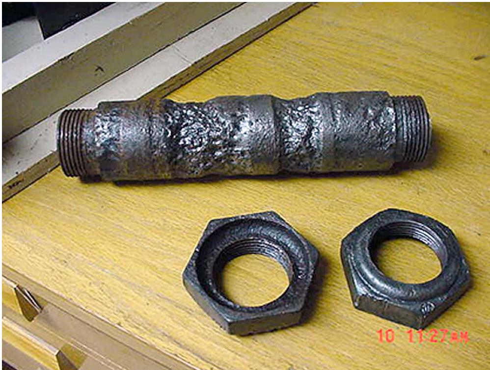
Figure 26. Heavily Corroded Pin; Section Loss Makes Removal Difficult
