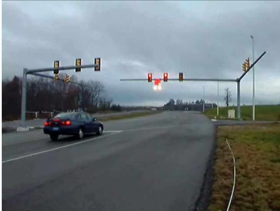
Figure 27. Lit LED stop sign along with fully functional strobes and TCLs.
