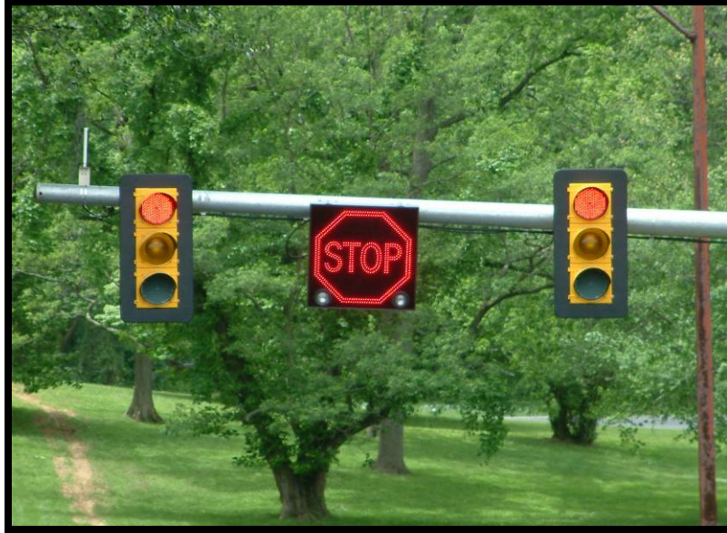
Figure 26. Lit LED stop sign. Unlit strobes are visible in the lower corners of the sign. The sign was completely opaque when unlit.
