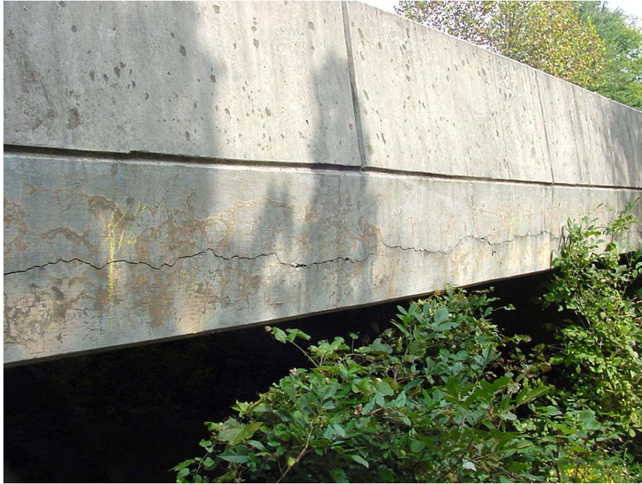
Figure 3. Cracks Along Length of Bridge
