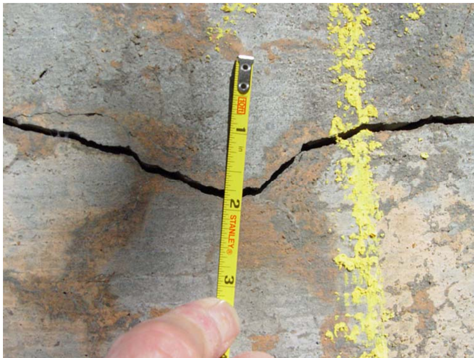
Figure 4. Cracks Can Be as Large as 0.25 In at Edge Surface of Slab
