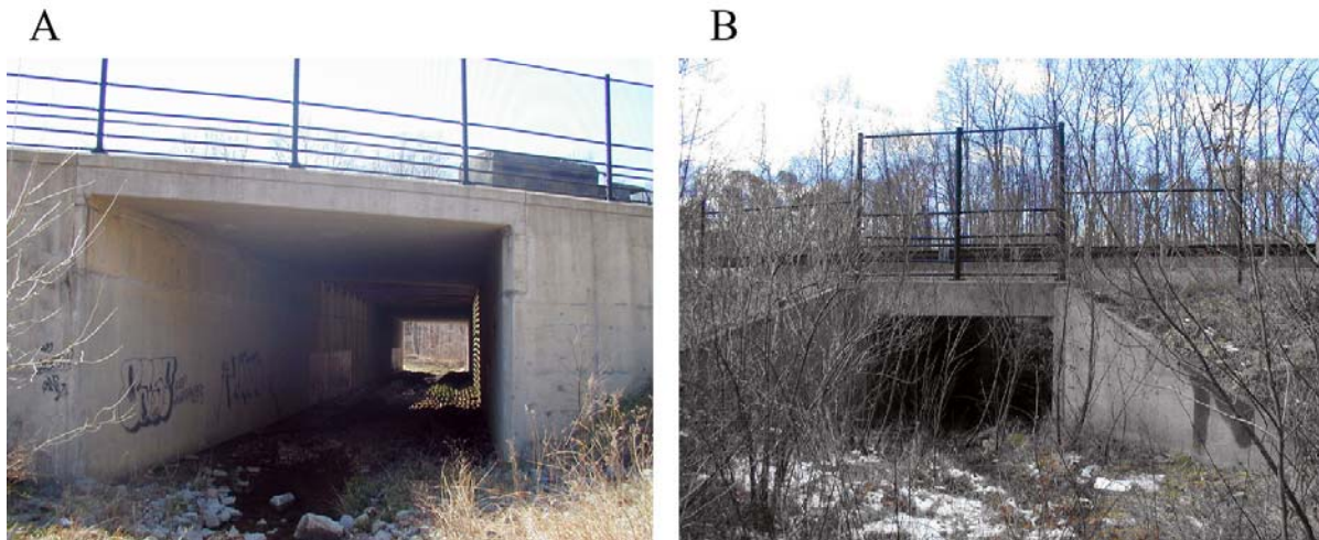
Figure 5. Sites 3A and 3B: Single-barrel Box Culverts 0.25 Mi Apart Beneath Fairfax County Parkway
