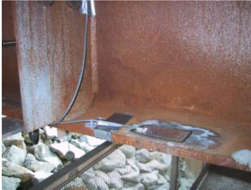
Figure 8. ER Strain Gauge on Steel Girder
