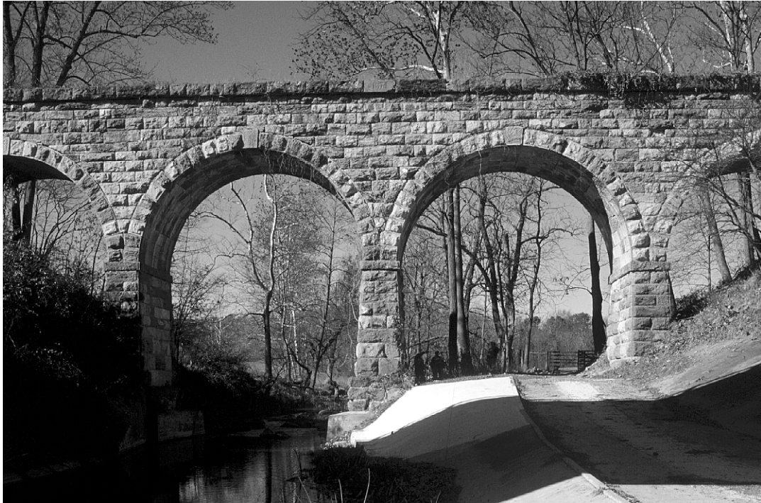
Figure 21. Solid Masonry Arch, Built in 1874 for the Valley Railroad (Now a well-known landmark within the right-of-way for I-81)
