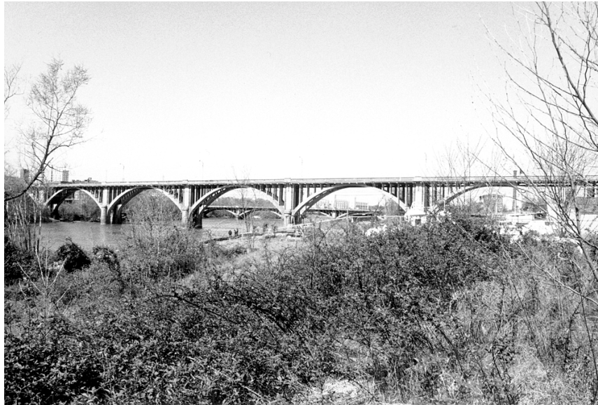
Figure 15. Open Spandrel Concrete Arch, a Luten Bridge Company Design Built in 1928 (City of Danville Structure No. 8006)
