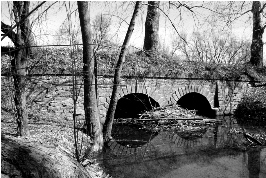
Figure 16. Solid Masonry Arch, Originally Built ca. 1835 as a Viaduct for the James River and Kanawha Canal (Nelson County Structure No. 6070)
