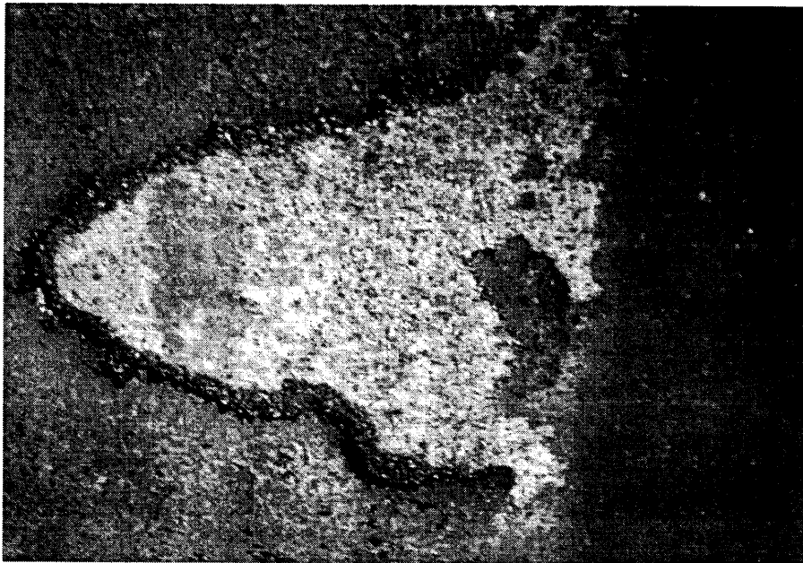
Figure 5. The same spall 1 year later.
