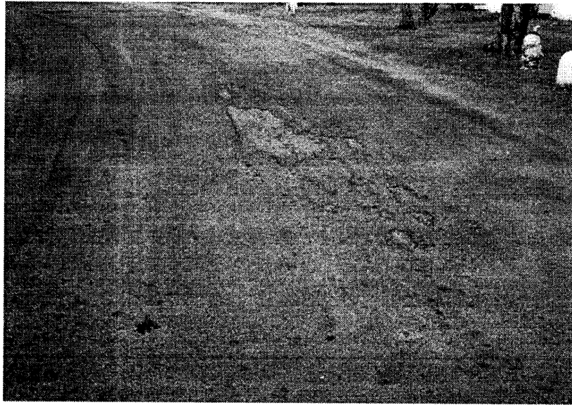
Figure 1. Spalled area in Clover Hills Subdivision.
