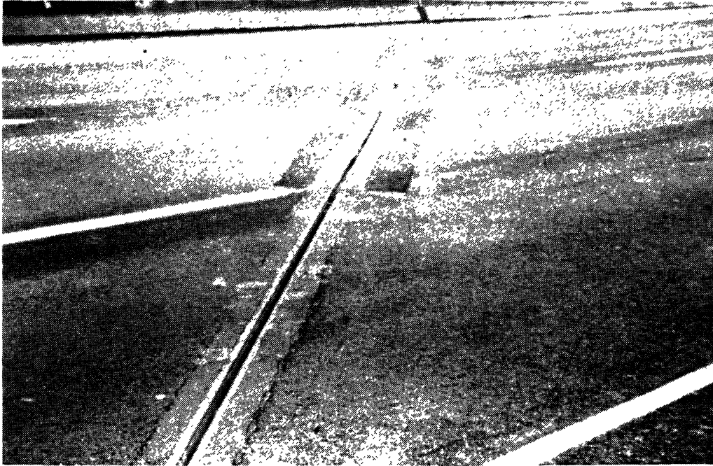
Figure 10. View of a Wabocrete FMV retrofit installation on a Capital Beltway bridge deck.
