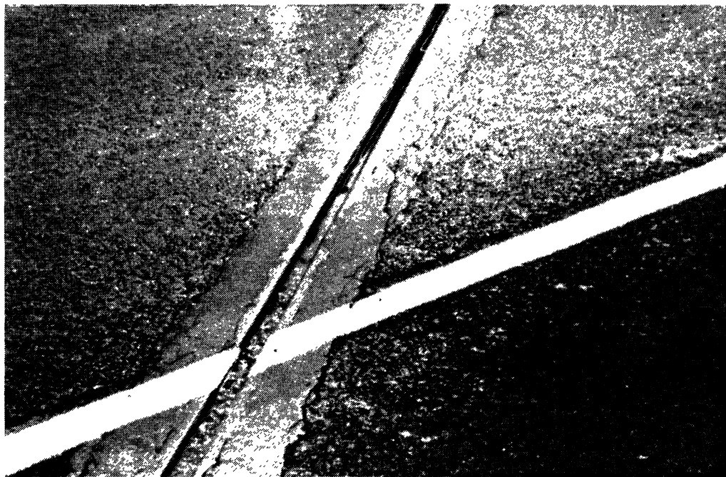
Figure 11. Separation at the interface between the joint and adjacent asphalt overlay.
