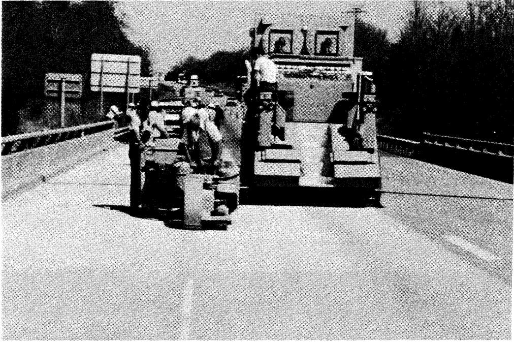
Figure C-1. Shotblast equipment cleans deck at rate of 12 yd 2 /min. Smaller unit removes paint lines (Rivanna River).
