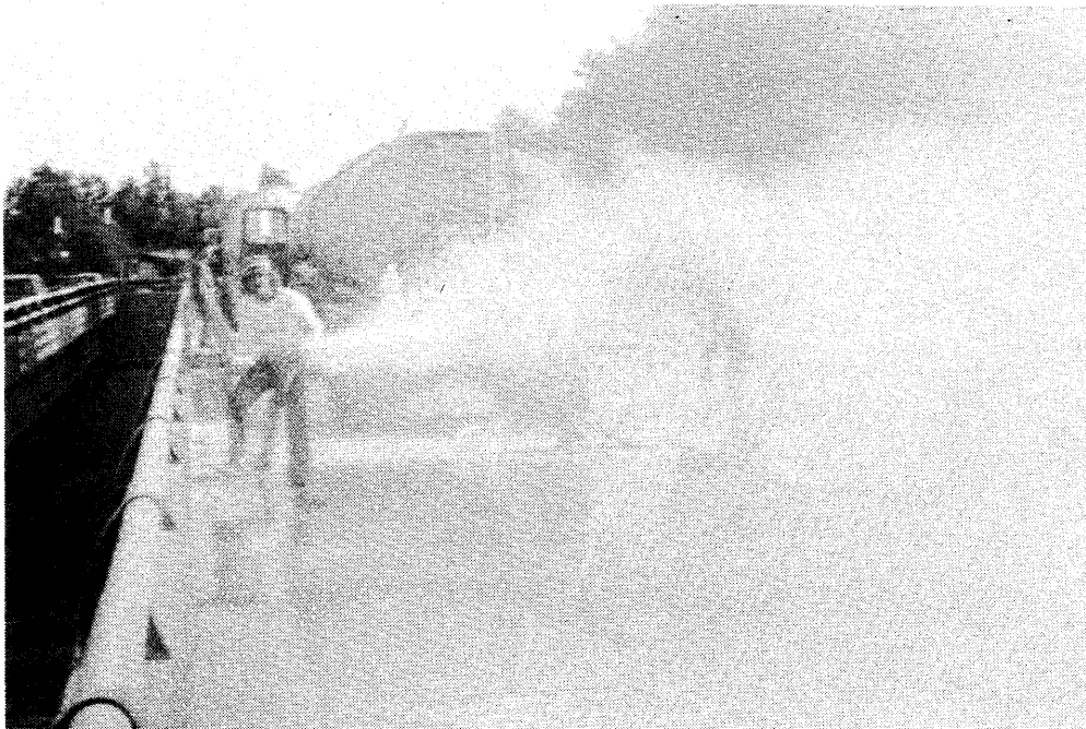
Figure E-3. Aggregate is blown into air with sandblasting equipment. (Rte. 123 over I-95).
