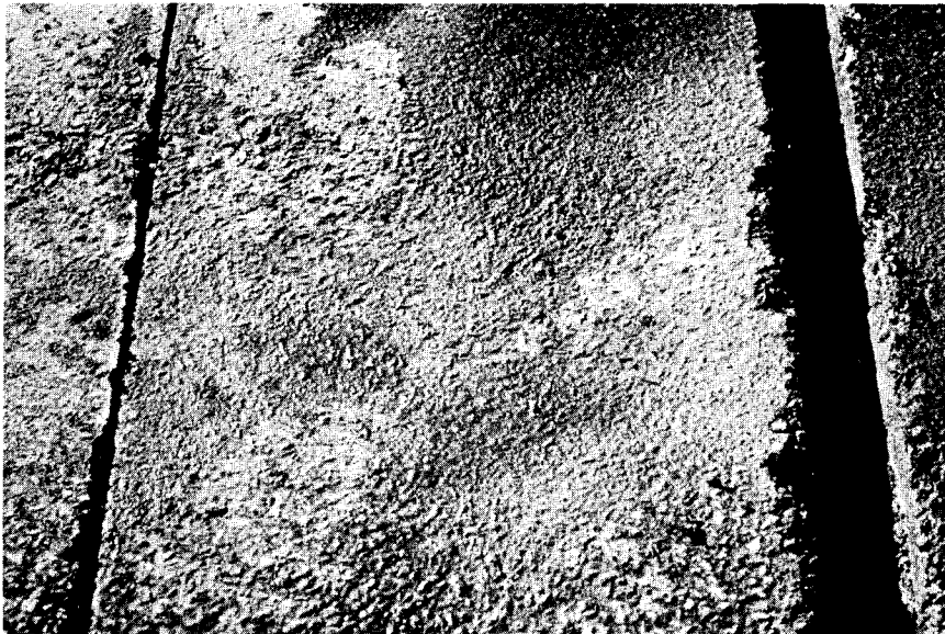
Figure 6. Comparison of saw cut for PVC loop (right) with typical saw cut.
