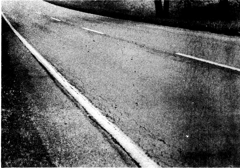
Figure 7. Edge cracking in Burlington glass fabric section of Route 29 at Charlottesville (SBL).
