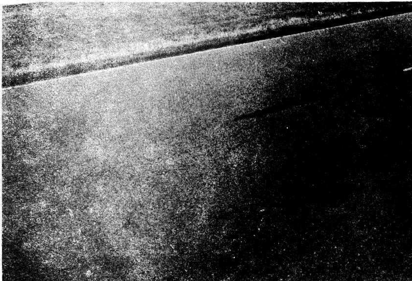
Figure 2. Cracking in Petromat section on Route 29 at Chatham.
