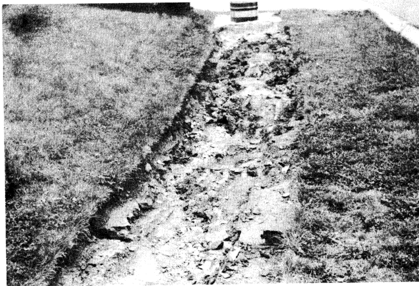
Figure 8. Test site showing erosion channel.
