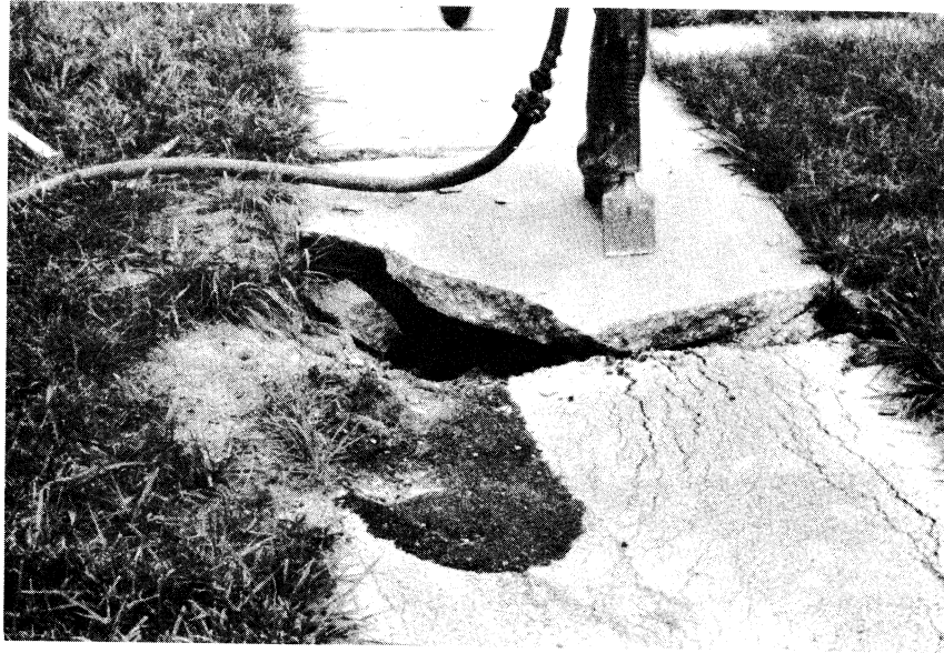
Figure 1. Severe sidewalk undermining.
