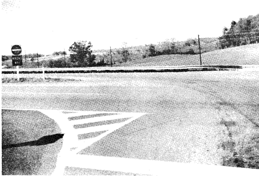
Figure 8. Junction of I-64 W exit ramp and Route 364 showing recently striped flare.
