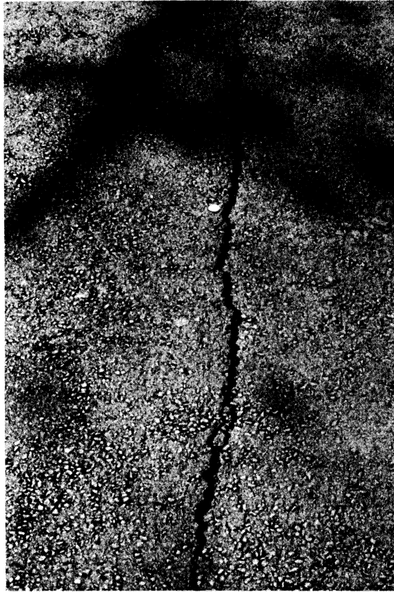
Figure 13. Crack in overlay on Henry County bridge.
