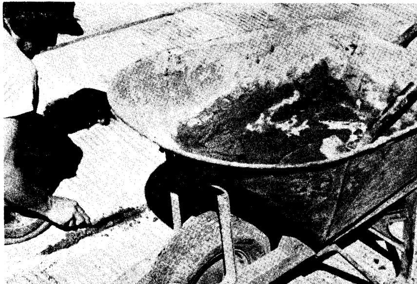
Figure 33. Nonshrink cement paste used to fill voids in precast parapets and the keyways between the tee beams was hand mixed at the bridge site.
