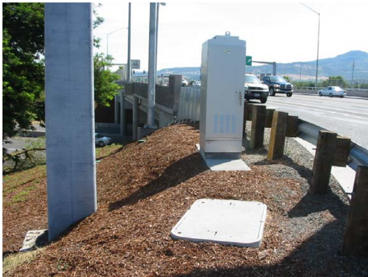
Figure 5.2: Signal control cabinet in Medford, OR
