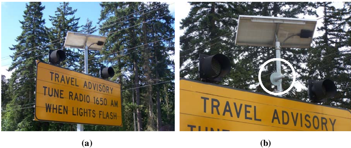
Figure 7.7: Setup for DCU2: (a) Beacon sign, (b) Installation location for antenna during testing
