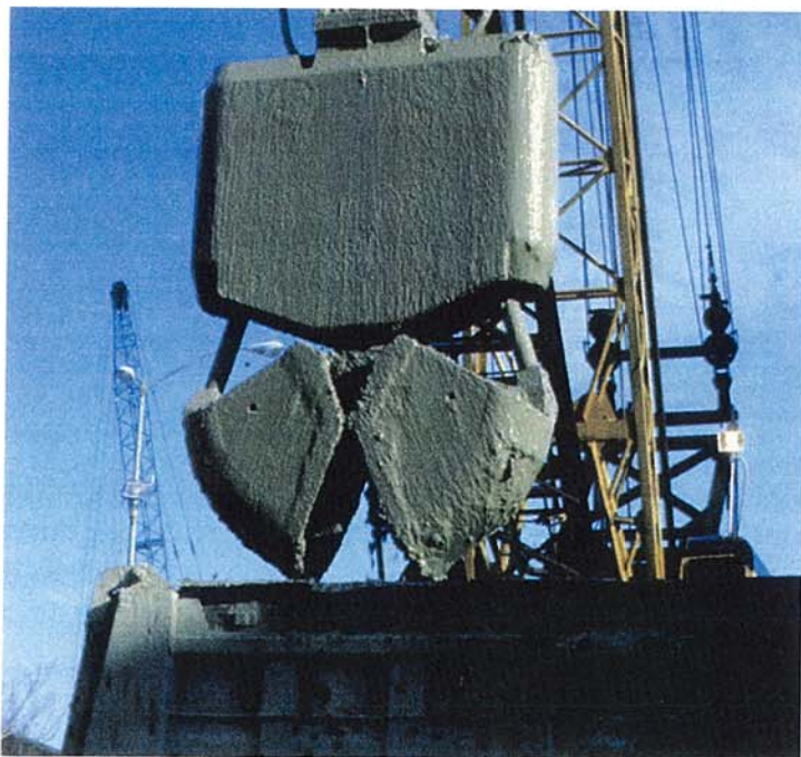
This specially designed clamshell was used to dig a narrow trench 40 feet deep. The slurry mix of clay and water was pumped into the trench as digging proceeded.
