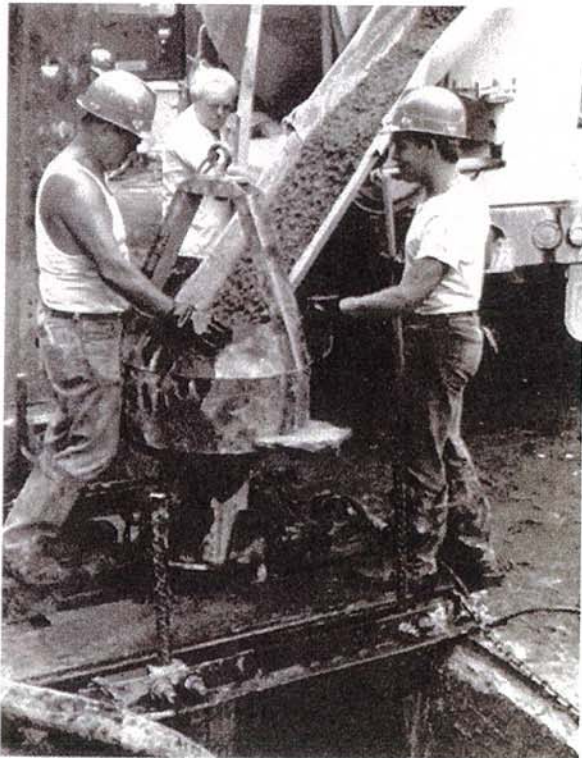
Next, concrete is piped to the bottom of the trench. As the concrete is added, the slurry rises to the top and is pumped off. It is then processed for re-use.
