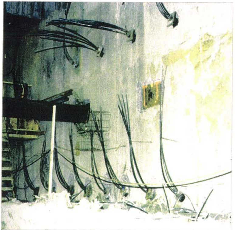
When the concrete has hardened, the tunnel is excavated and the walls are anchored to the soils outside the tunnel. Anchors consist of nests of reinforcing bars that are spread apart outside and then stabilized by injecting a grout.
