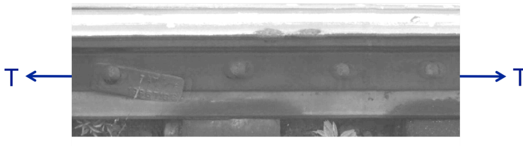
A: Original Image Switch Point Bolts
