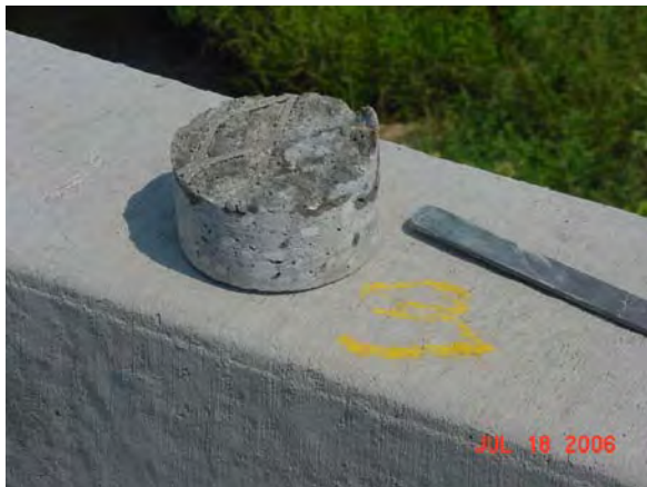
Figure 10: Core 3 – only one with anode imbedded in concrete.
