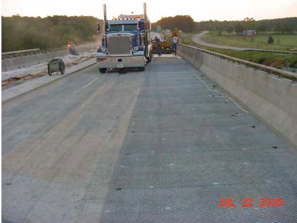
Figure 4: Anode laid out ready for concrete. Note: White spots are plastic anchors to hold sheet in place during concrete placement foreground.
