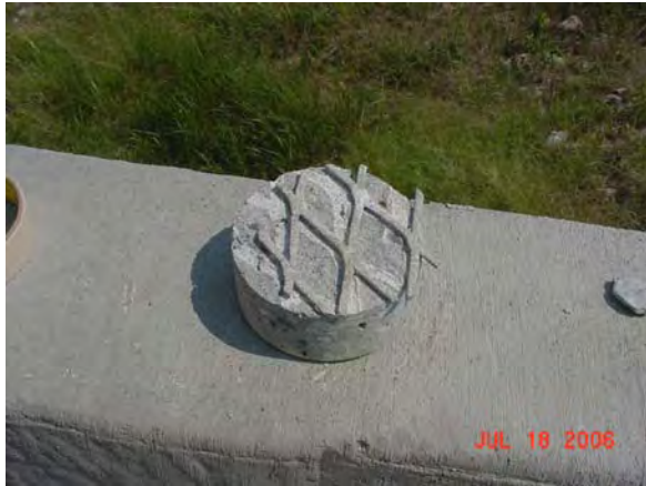
Figure 8: Core #1 –anode disbonded.
