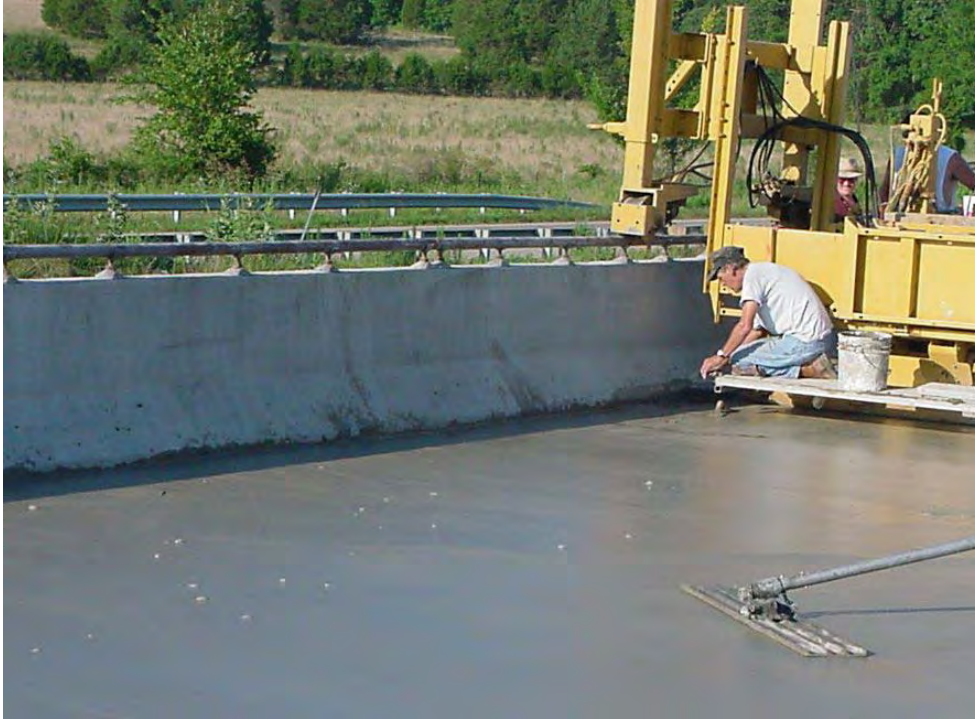
Figure 6: Gas bubbles from cement reacting with Al-Zn-In coating on anode appeared before final finishing of the overlay.
