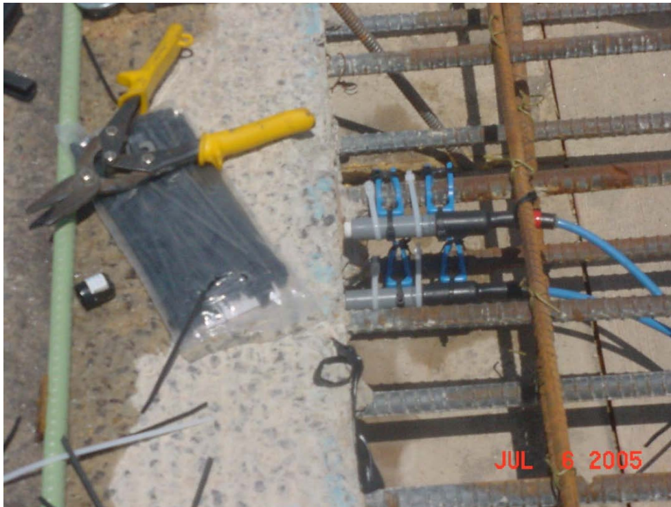
Figure 1: Silver/Silver Chloride Half Cells, one at level of top rebar and one at bottom rebar.
