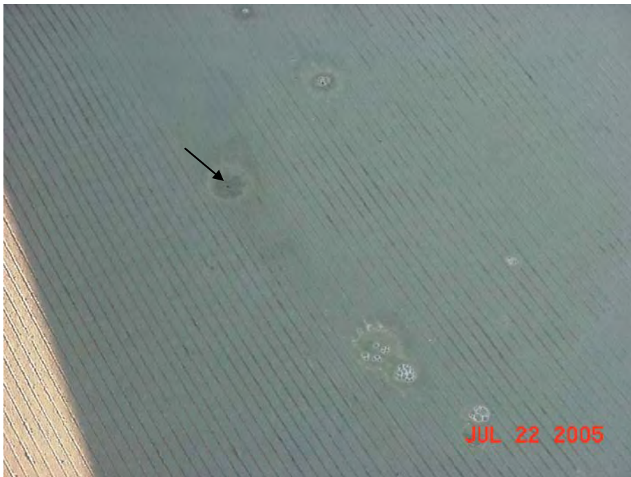
Figure 7: Close up of gas bubbles coming up after surface textured. Note: one on left in middle has popped and a black pin hole can be seen in its center. Does it go all the way through the 2" thick overlay?
