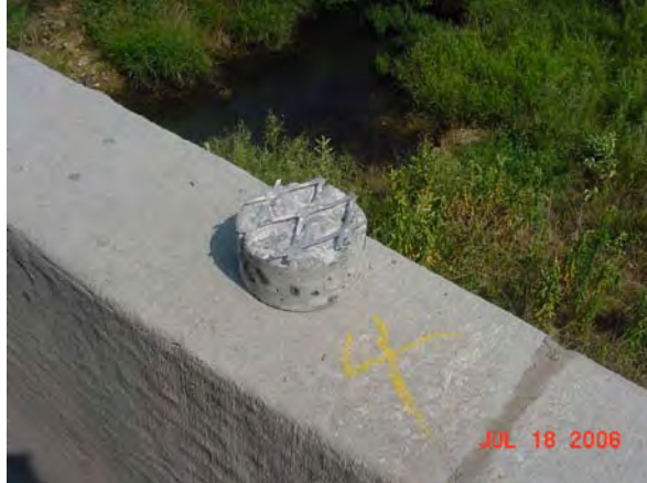
Figure 11: Core 4 – anode disbonded.
