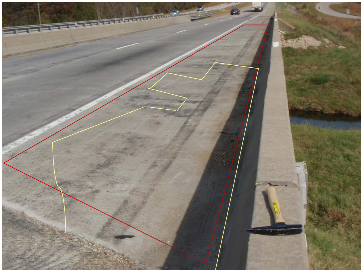
Figure 12: October 2010 photo of concrete deck overlay above the Al-Zn-In anode (outlined in red), five years after installed. There are few cracks and no spalling on the surface but 46% of the concrete overlay is debonded over the anode (outlined in yellow). See maps in Appendix B for additional debonded areas.
